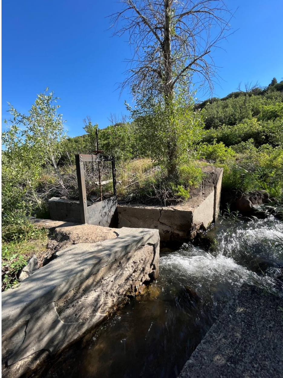
Head Gate Diversion, Right Bank Battlement Creek Concrete Spalling Either Side of Head Gate
