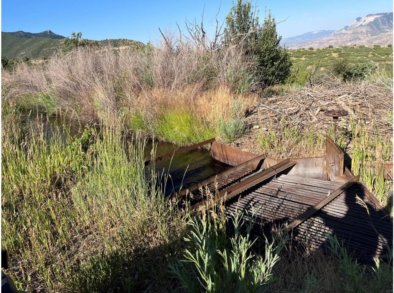
Splitter Box at End of Open Ditch End of Buried Pipe Approximately 30' u/s
