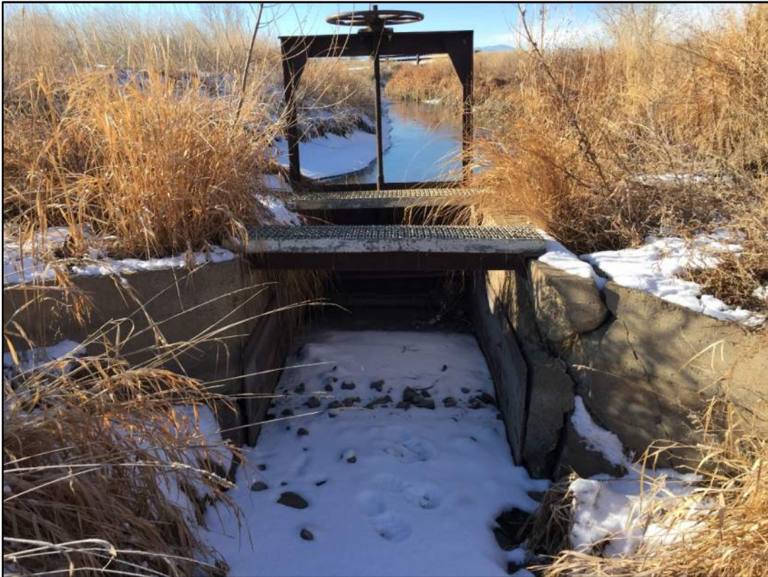
Photo 2: Smith and Emmons Ditch Headgate - Detail
