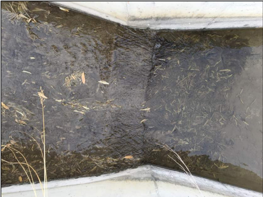
Photo 6: Smith and Emmons Ditch Measuring Flume - Throat Detail
