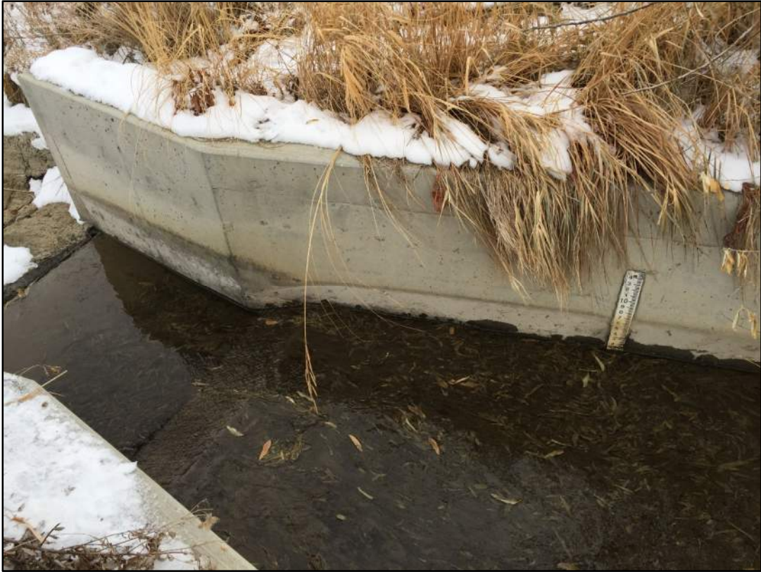
Photo 5: Smith and Emmons Ditch Measuring Flume
