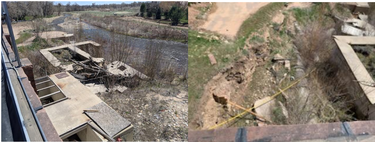
Figure 7 Debris to be removed
