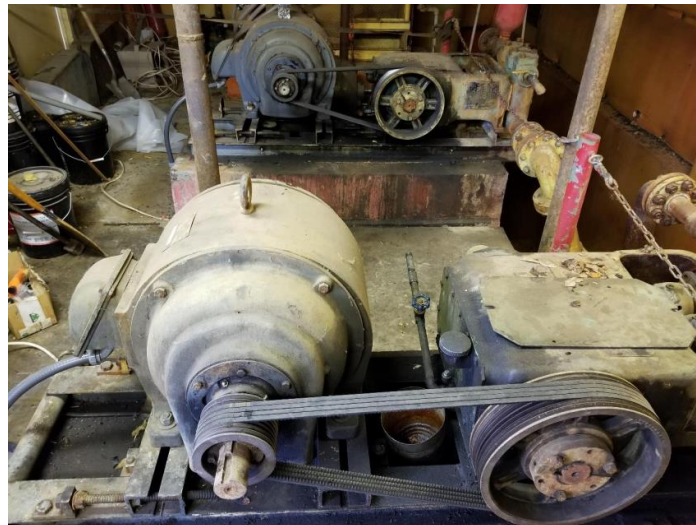
Figure 2. Existing Pump Need at Dolores River
