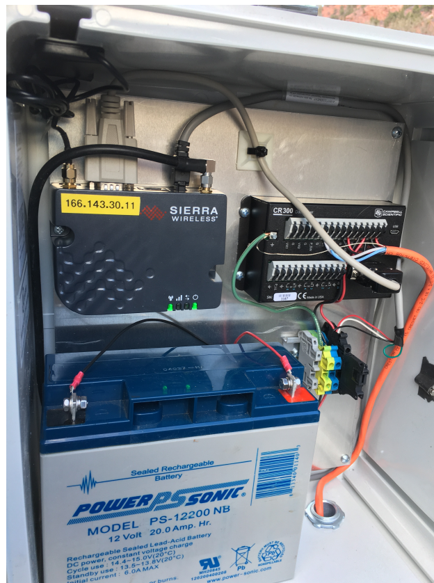
Figure 2. Typical instrumentation wiring and housing.
