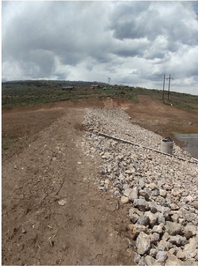
Figure 1. Von Springs #1 – Low-Level Outlet with Grade Beam and Service Spillway Standpipe
