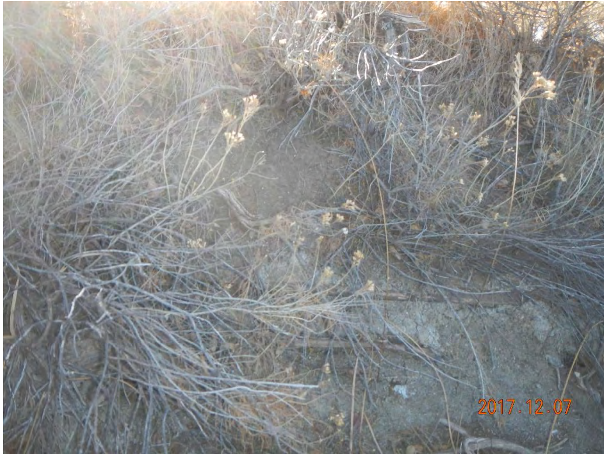
03_Upstream Slope, roots
