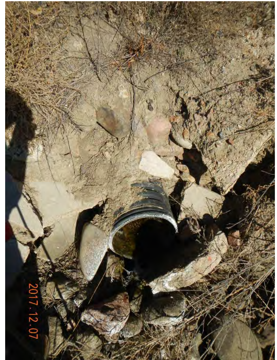
12_Seepage, previous failure
