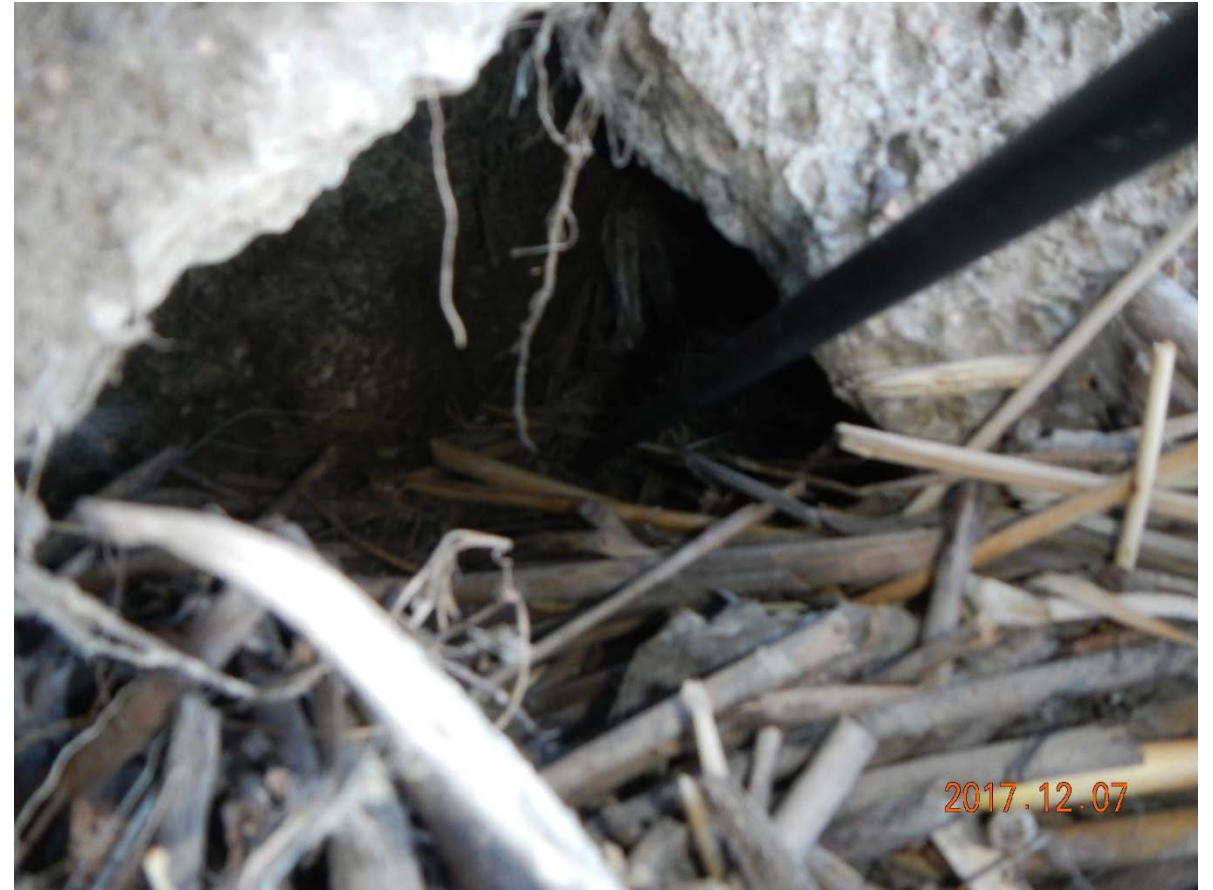
06_Upstream Slope, previous failure location
