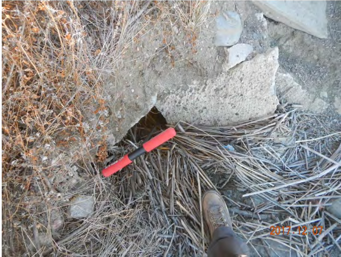
05_Upstream Slope, previous failure location
