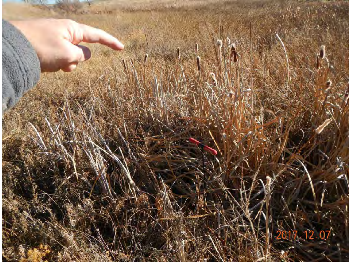
19_Seepage area left of outlet
