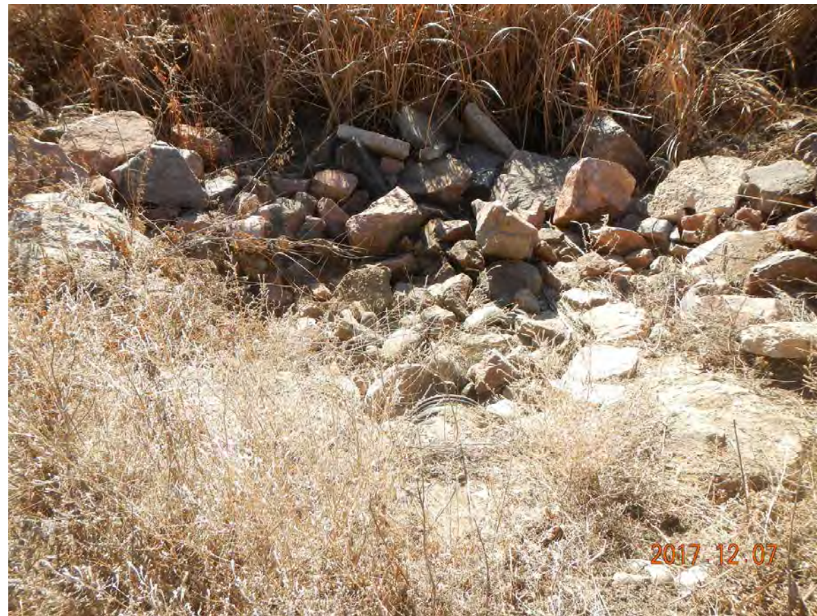
14_Seepage, previous failure
