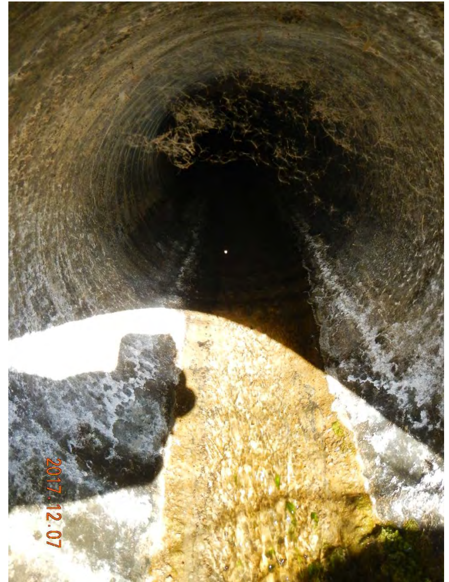
15_Seepage, previous failure
