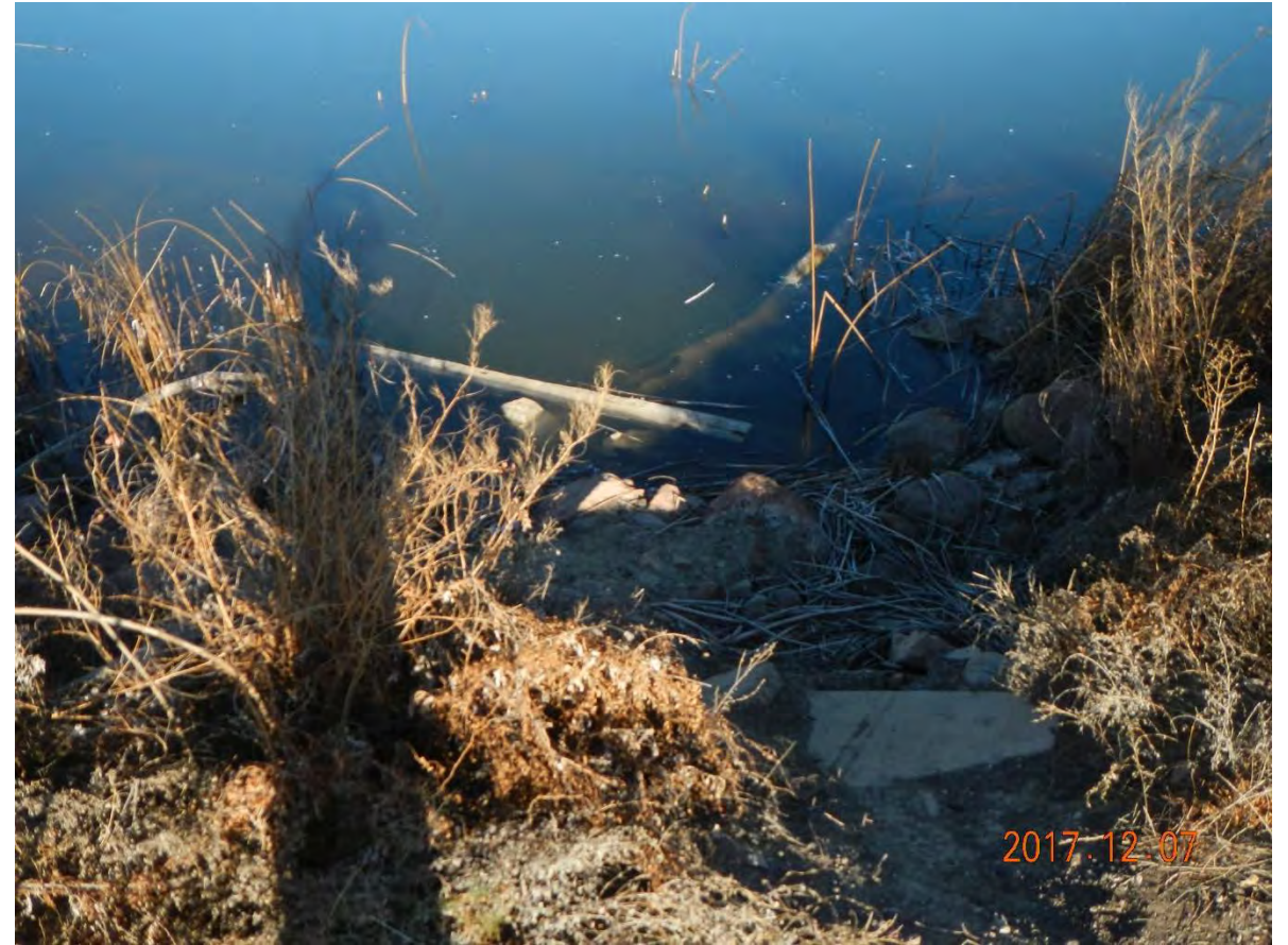
04_Upstream Slope, previous failure
