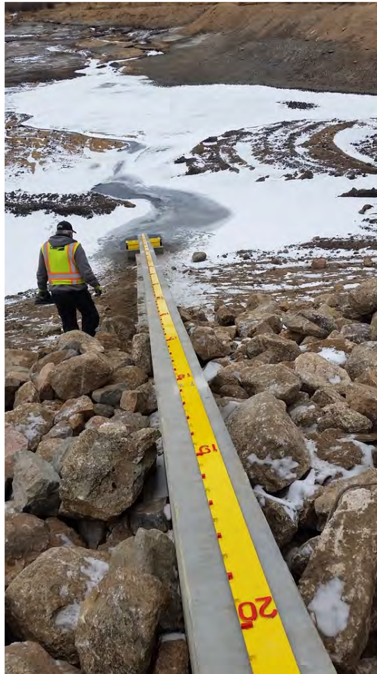
Figure 4. Harris Park #2 – Low-Level Outlet with Grade Beam and Steel Staff Gage
