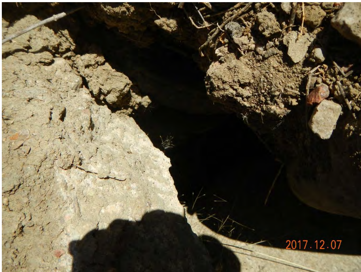
13_Seepage, previous failure
