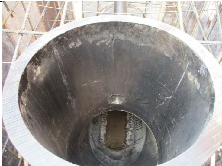
Photo 4. HDPE Pipe is level and must be cut/beveled to accommodate gate as shown in profile in detail B, sheet 12. Air vent penetration is visible in the back of the pipe.
