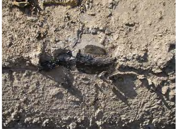
Photo 4. Close-up view of old pipe exterior - seam along side of pipe appeared discontinuous - the section of pipe upstream likely was turned over, with the seam located beneath
