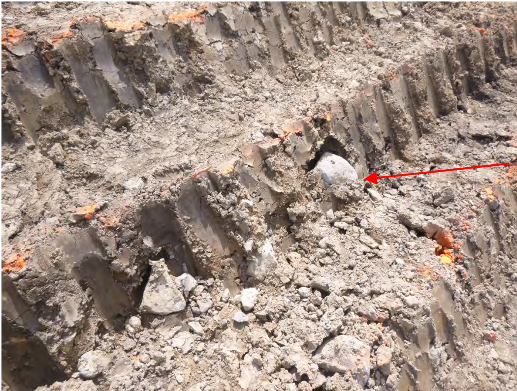
Example of oversized particle in bench that should be removed prior to fill placement. Void needs treatment prior to backfill.
