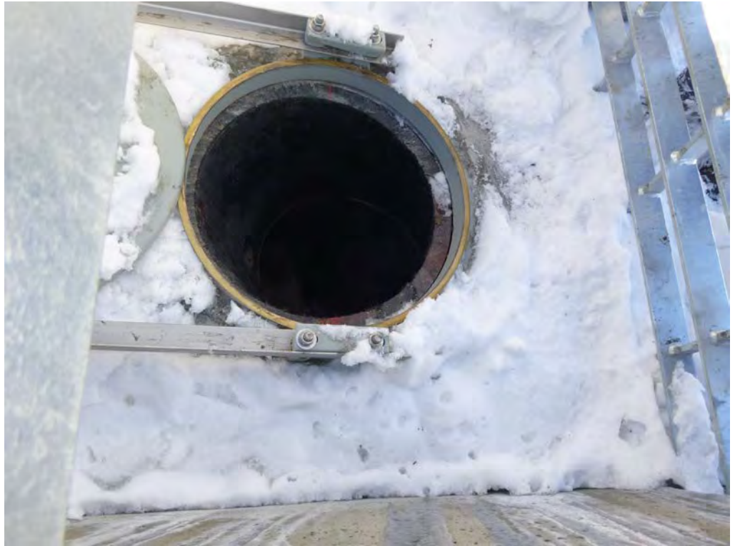
Outlet gate in full open position during exercise.
