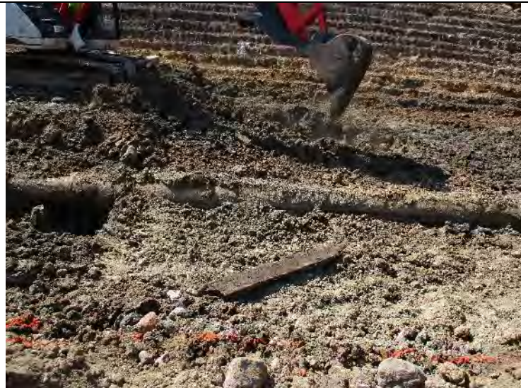
Photo 6. Formwork left in place from original construction
