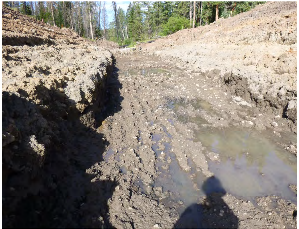
Close-up of typical area of standing water; location is near Sta 1+20 for the outlet sand diaphragm.
