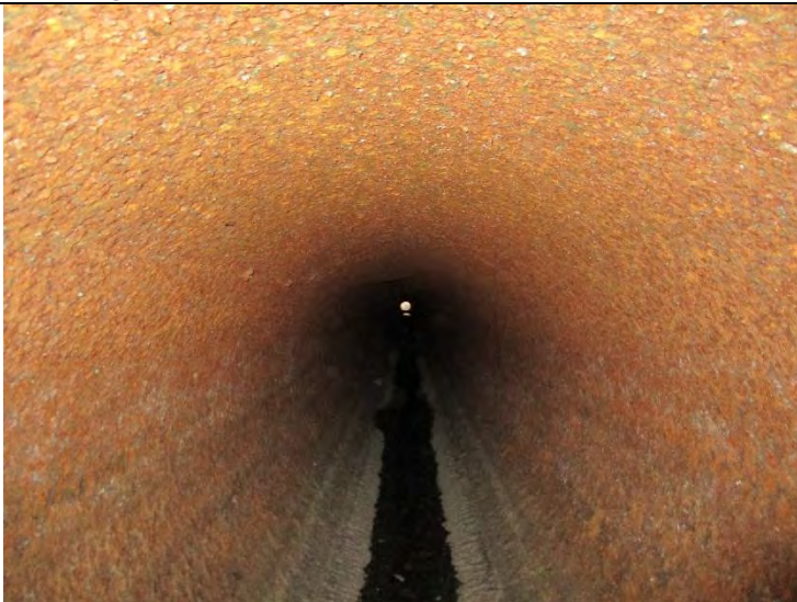
Photo 5. Interior view of old pipe - surprisingly good condition
