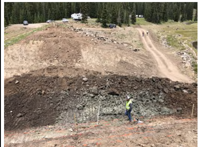
Photo 4. View of grey clay pocket on the east side of the breach excavation looking west towards campground.
