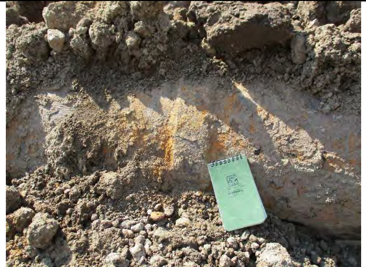
Photo 2. Old pipe joint
