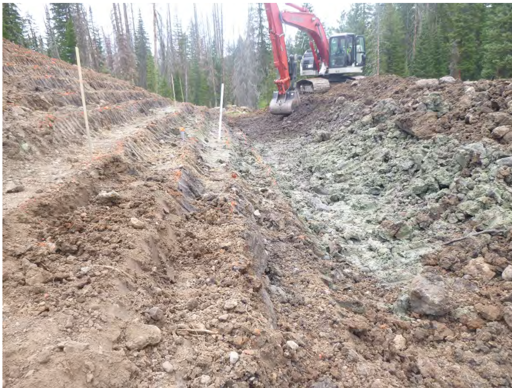
View looking downstream along left sideslope of breach with pre-formed benches. Blue clay can be seen in foreground.
