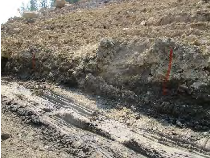
Photo 3. One of two soft spots identified during first proof roll.
