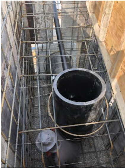
Photo 1. Close-up view of inlet structure reinforcing steel. Note gap in horizontal bars above the ConSy staff member.
