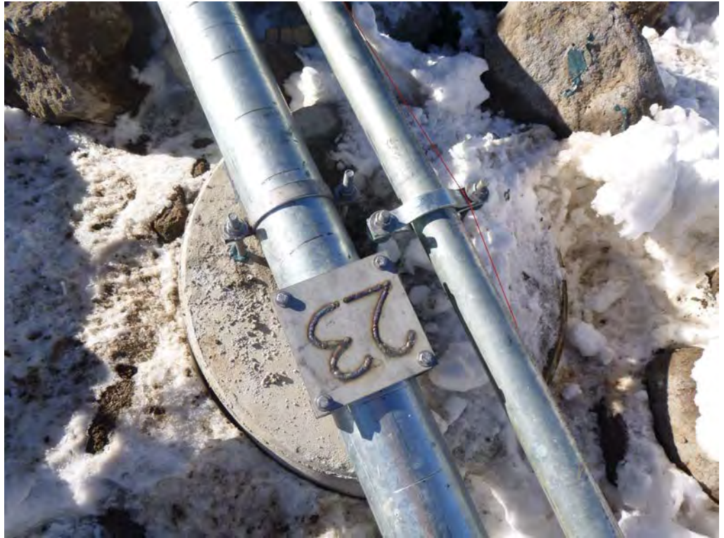
Typical support pier with air vent and gate stem clamps.
