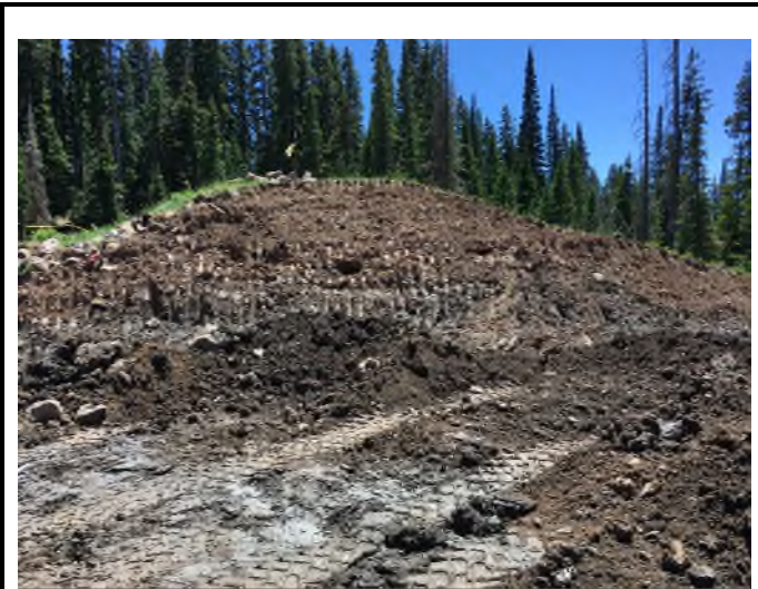
Photo 3. View of breach and outlet prior to start of project. Photo taken on July 13, 2020.
