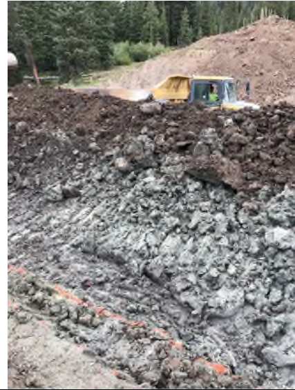
Photo 2. Close-up of blue clay pocket on the east side of the breach excavation
