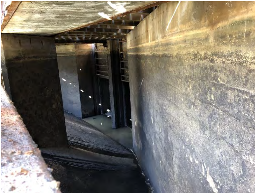
Figure 2.4.2. Penstock Gates in Turbine Forebay
