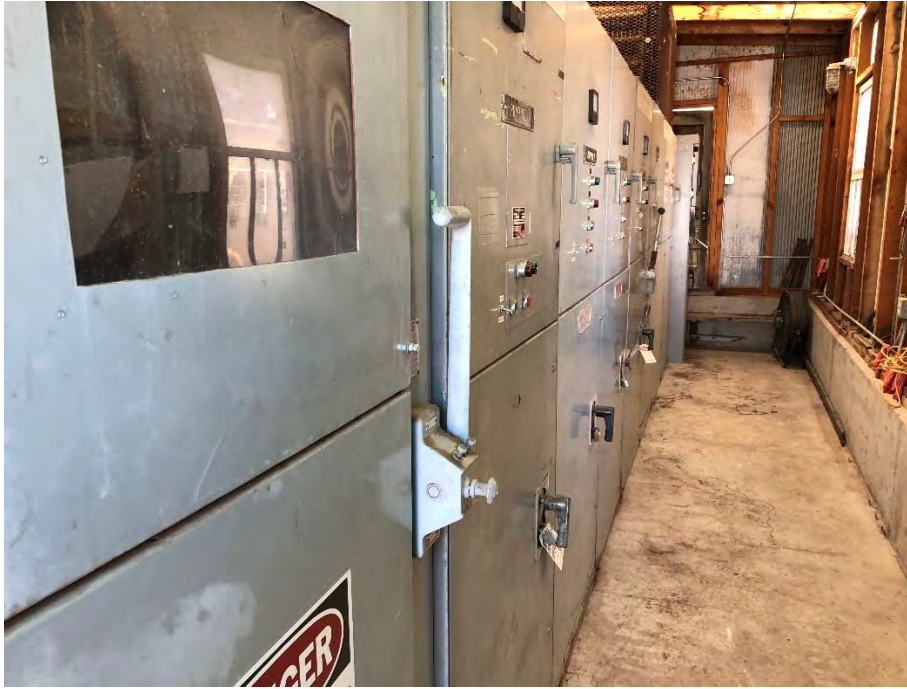
Figure 2.2.3 Pump Station Control Room
