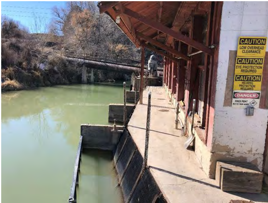
Figure 2.2.1 Pump Station Exterior Configuration
