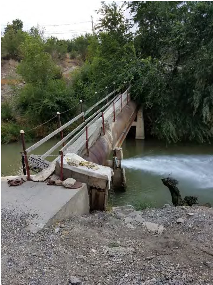
Figure 2.3.1. Power Canal Overshot
