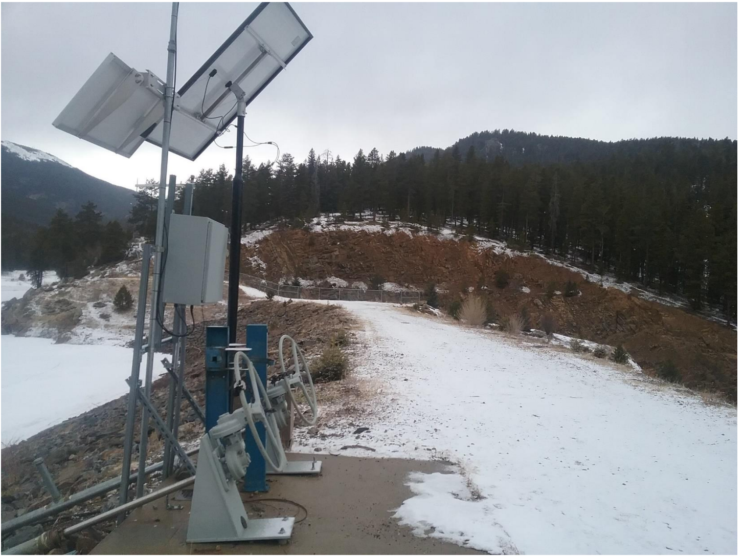
Figure 5: Photo of Upper Beaver Brook Reservoir Gate Controls
