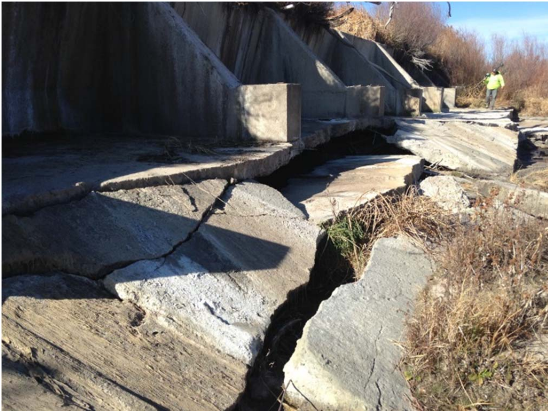
Fig. 4: Collapse of downstream floor slab, diagonal section.
