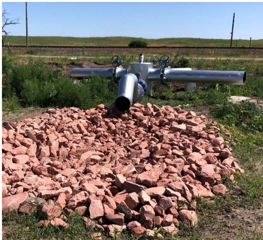
Picture 1- Three-way valve tree and flowmeter
