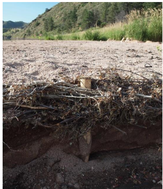
Figure 8. Post-storm damage on recently installed bank treatments at Seaman Reservoir.
