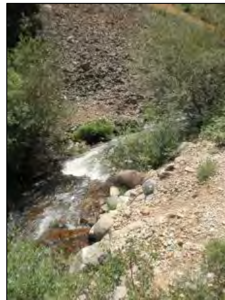
Photo 12. Impacts from road encroachment - looking downstream.
