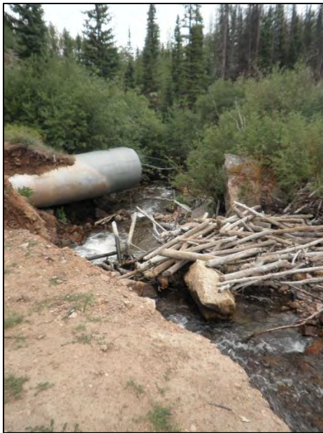
Photo 33. Impact Site No. A6, Rat Creek. Erosion impacts from culvert and road encroachment.
