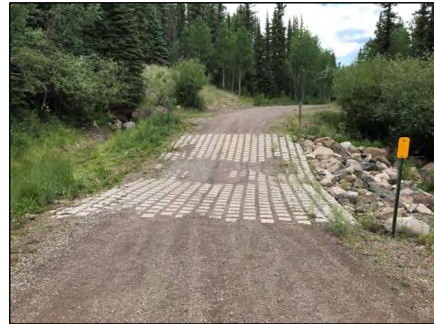
Photo 26. Impacts from road crossing and culvert.
