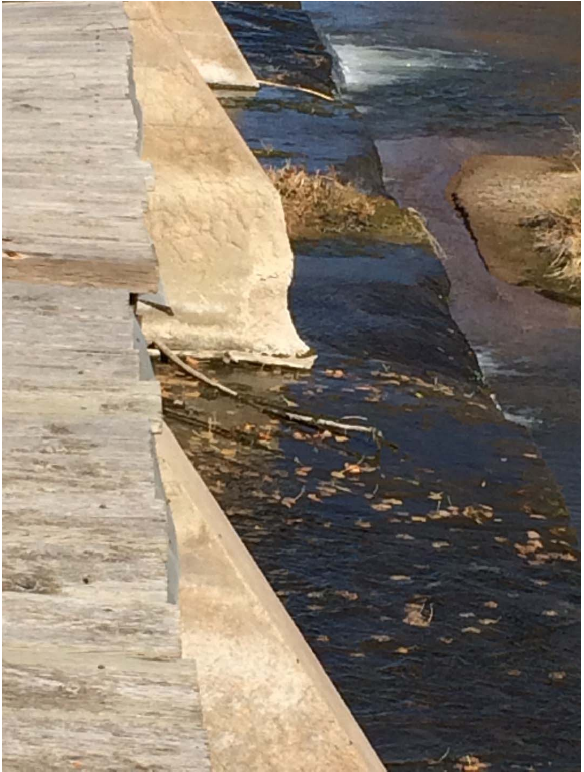
PHOTO 4 – DIVERSION STRUCTURE DETERIORATED CONCRETE
