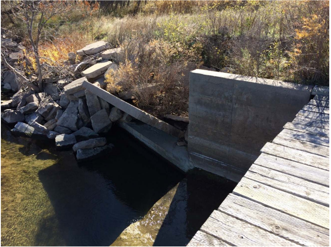
PHOTO 3 - RIGHT (SOUTH) ABUTMENT BLOWOUT
