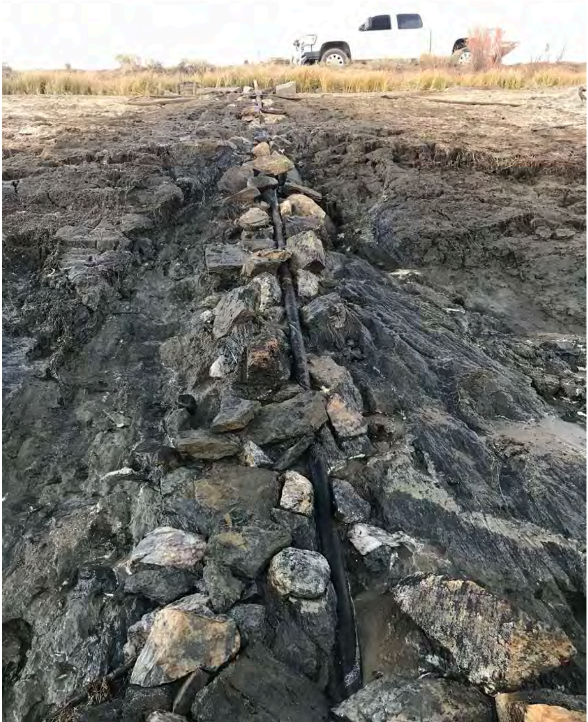
63. View of the air vent pipe near the low-level outlet where the staff gauge will be installed.
