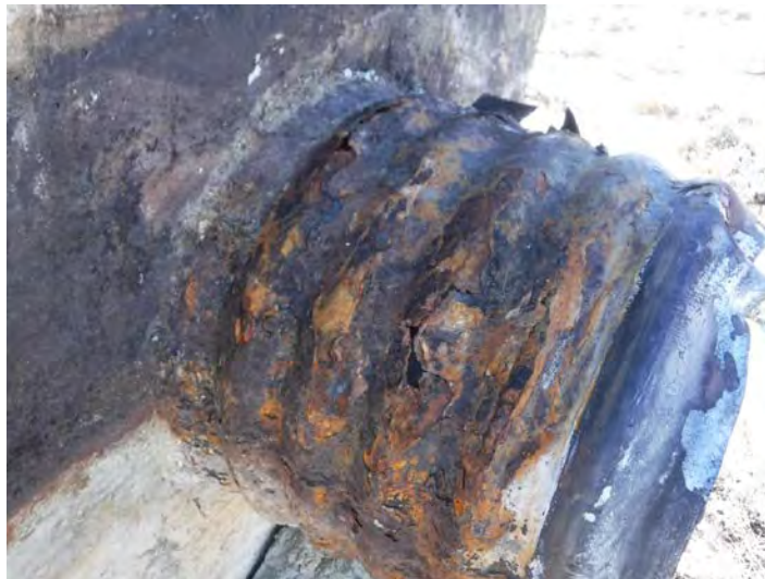
Photo 7 Corroded pipe segment just upstream of the old headwall; note silver appearance of CMP just upstream (right side of photo)
