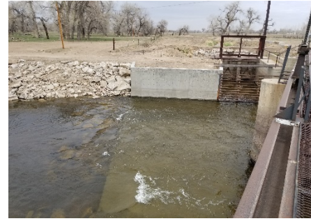
Figure 6 - Lupton Bottom Ditch headgate.
