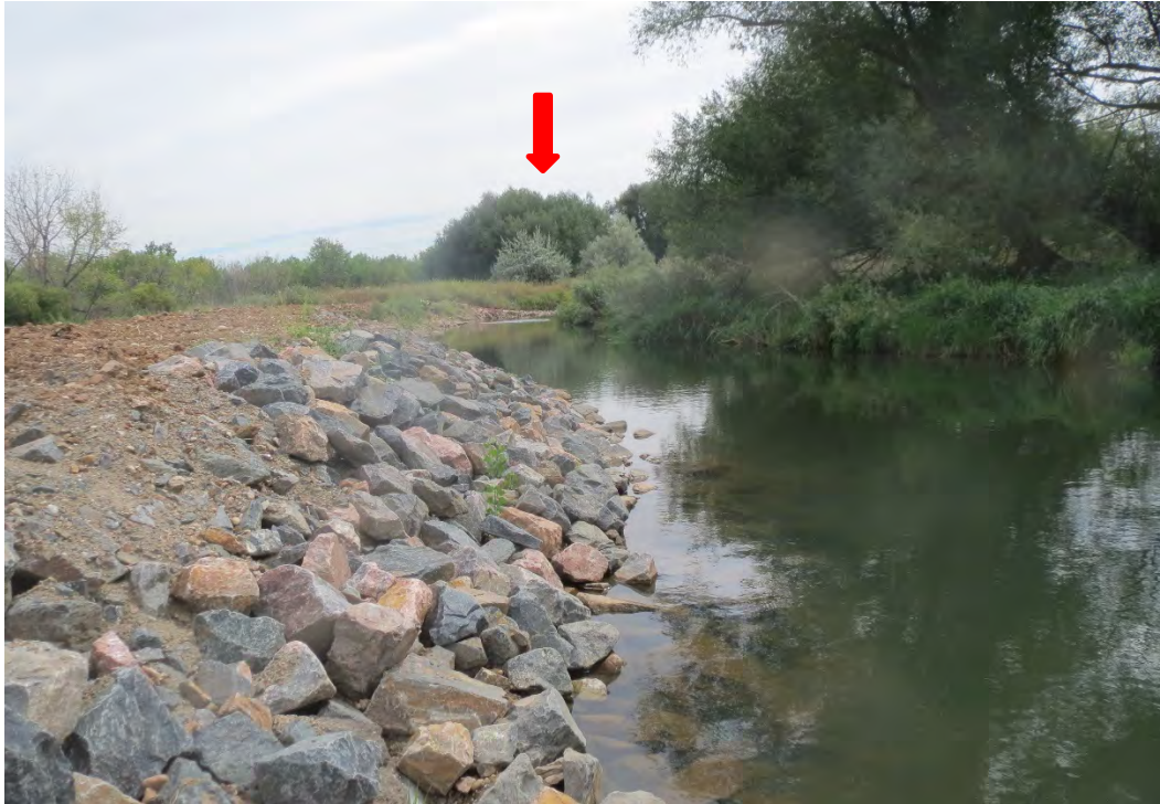
Photo 20. Prior to restoration, the temporary riprap berm provides poor habitat. Creek dimensions created an entrenched channel. View facing downstream September 7, 2016.
