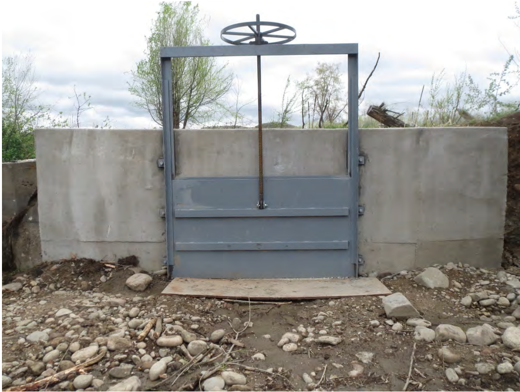
Photo 2. New Green Ditch headgate.
