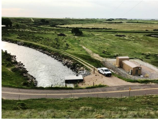
Pump Station No. 1 at the outlet of North Sterling Reservoir. This is 1 of 4 pump stations to move the water 37 miles and lift it 750 feet in elevation.
