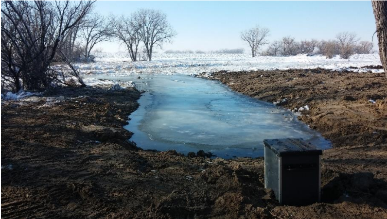
Figure 4. One of the Agri Drain stoplog inline water control structures installed at DPG Prewitt project near Merino, Colorado. The structure facilitates management of water levels to promote growth of annual wetland plants and preclude monotypic cattail stands.
