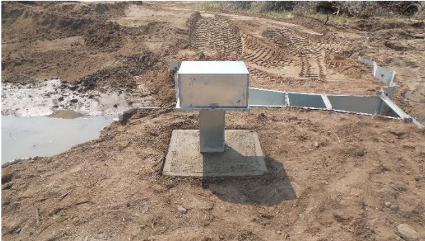
Figure 8. Installed Parshall flume below the water control structure for the Prewitt State Wildlife Area wetland enhancement project near Merino, Colorado.
