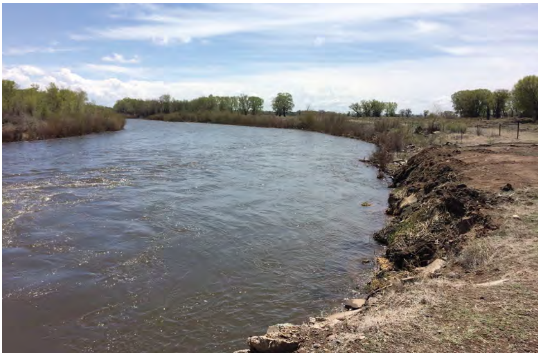
Figure 6: Example of steep, eroding streambanks in the Project Area
