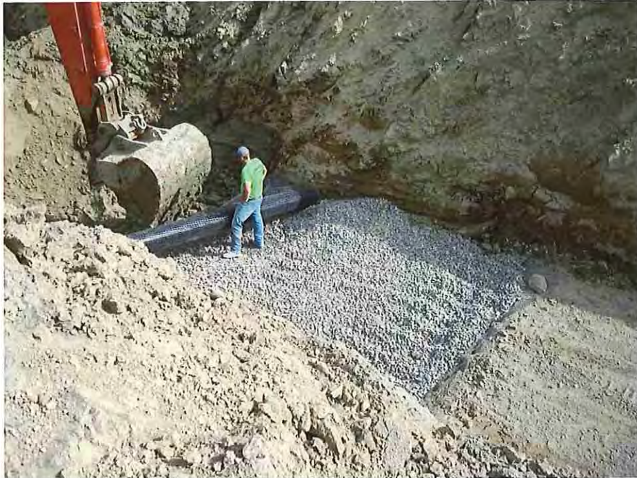
Photo #11: September 21, 2016 – Installation of the stabilization rock and geogrid in the toe-drain excavation between stations 2+50 to 3+25 +/- . Stabilization rock was a 1-1/2" crushed rock and a 2-foot thick layer of rock was placed above the soft subgrade material. Geogrid was placed in the middle of the 2-foot thick rock layer.
