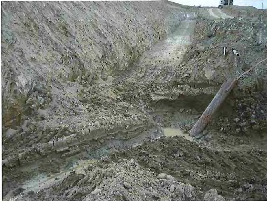
Photo #9: September 20, 2016 – The toe-drain excavation encountered wet and soft subgrade conditions between toe-drain stations 2+50 to 3+25 +/- . Stabilization rock and geogrid would be used to stabilize this area for placement of the filter sand, drain gravel and toe-drain pipe. Photo shows contractor pumping out the ground water/seepage water.
