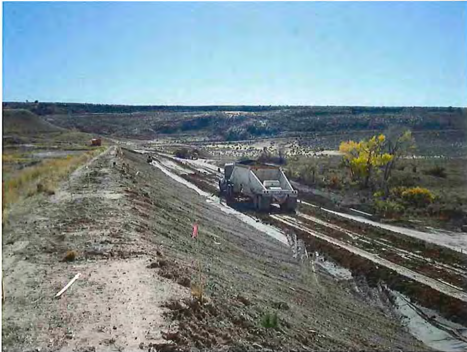
Photo #29: October 27, 2016 – Embankment fill operations in relation to the existing dam crest.
