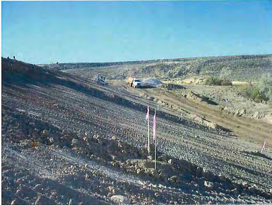
Photo #5: September 9, 2016 – Photo looking at the 2-ft deep over-excavation of the dam slope (Sta. 2+89 to 3+79). This area corresponds to the area of the dam that developed the downstream crack(s).
