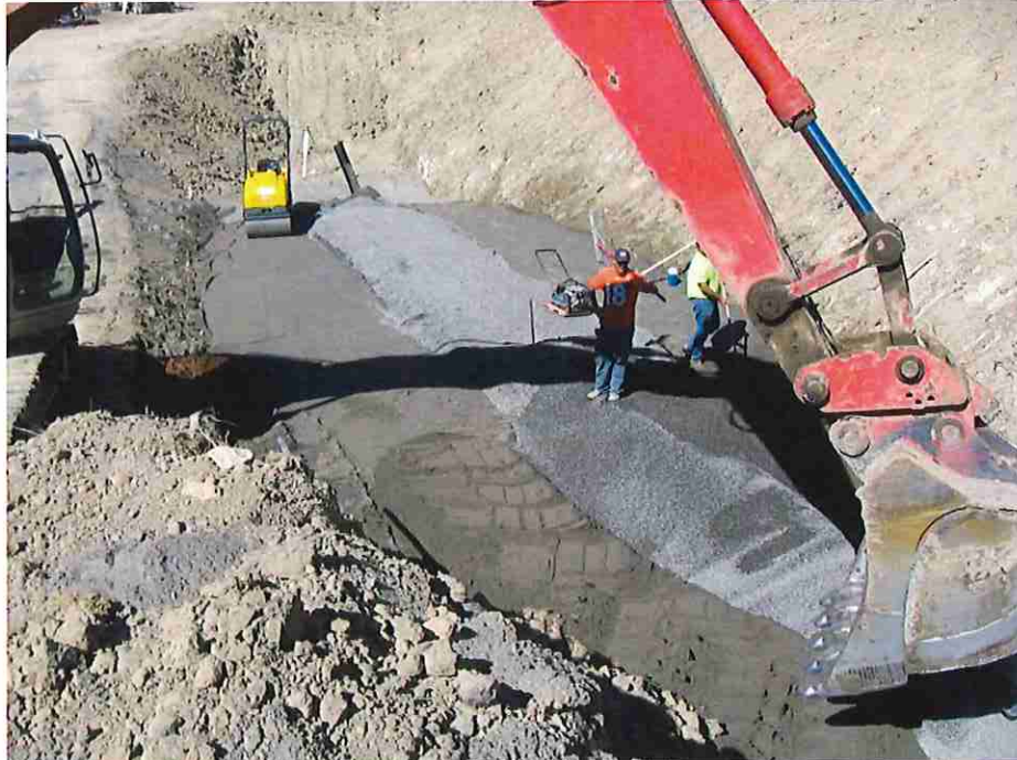
Photo #16: September 27, 2016 – Photo shows the south toe-drain being installed. Filter sand and drain gravel encapsulate the 8-inch diameter HDPE toe-drain pipe. The toe-drain pipe can be seen in this photo to the right of the smooth drum roller.
