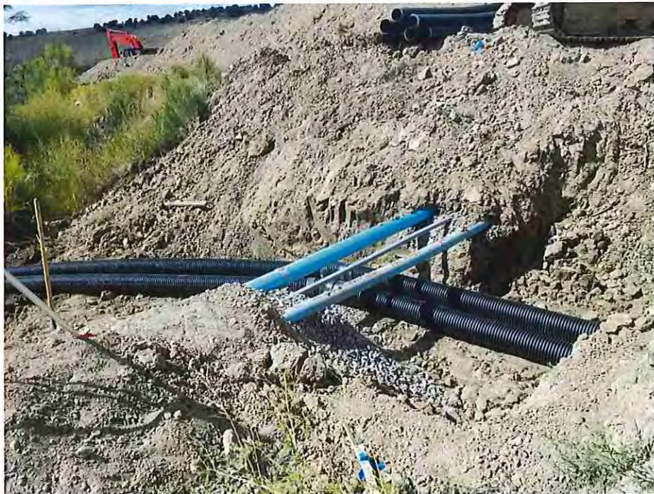
Photo #14: September 22, 2016 – North and south toe-drain outfall pipes daylighting out into the drainage. Pipes shown above the toe-drain pipes are the City's 4-inch domestic water supply line, the future 6-inch domestic water supply line and a 2-inch electrical conduit.
