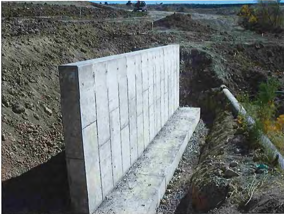
Photo #27: October 20, 2016 – Completed concrete retaining wall. Embankment fill will be placed and compacted around the wall.
