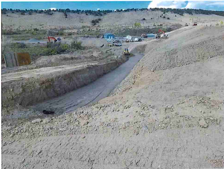
Photo #18: September 30, 2016 – South toe-drain pipe installed and encapsulated in the filter sand and drain gravel. Ready for embankment fill to be placed on top of the filter sand.
