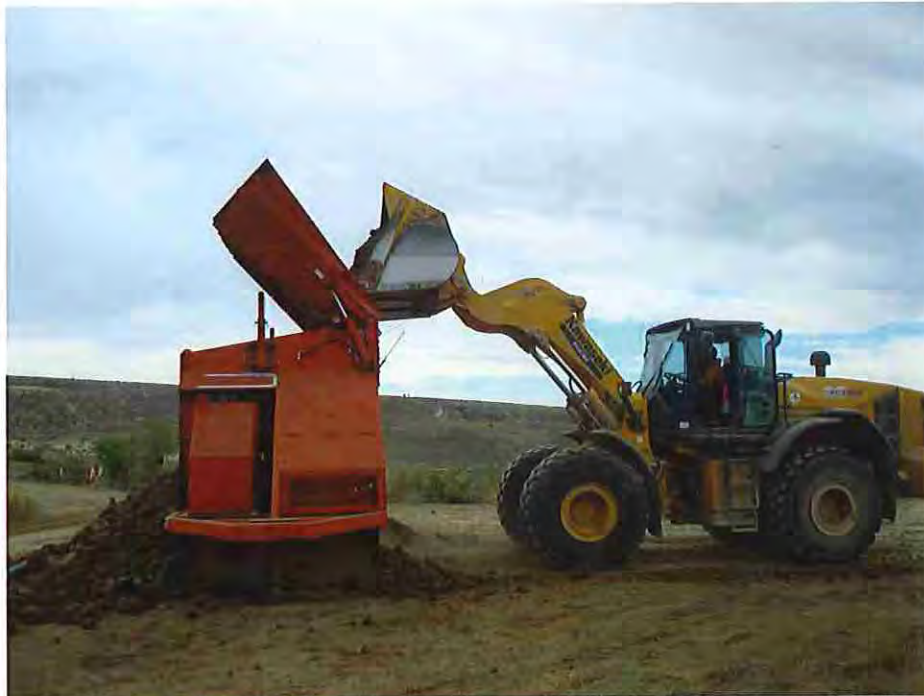
Photo #10: September 21, 2016 – Contractor processing the proposed embankment fill to get rid of rocks that are larger than 4-inches per specification.
