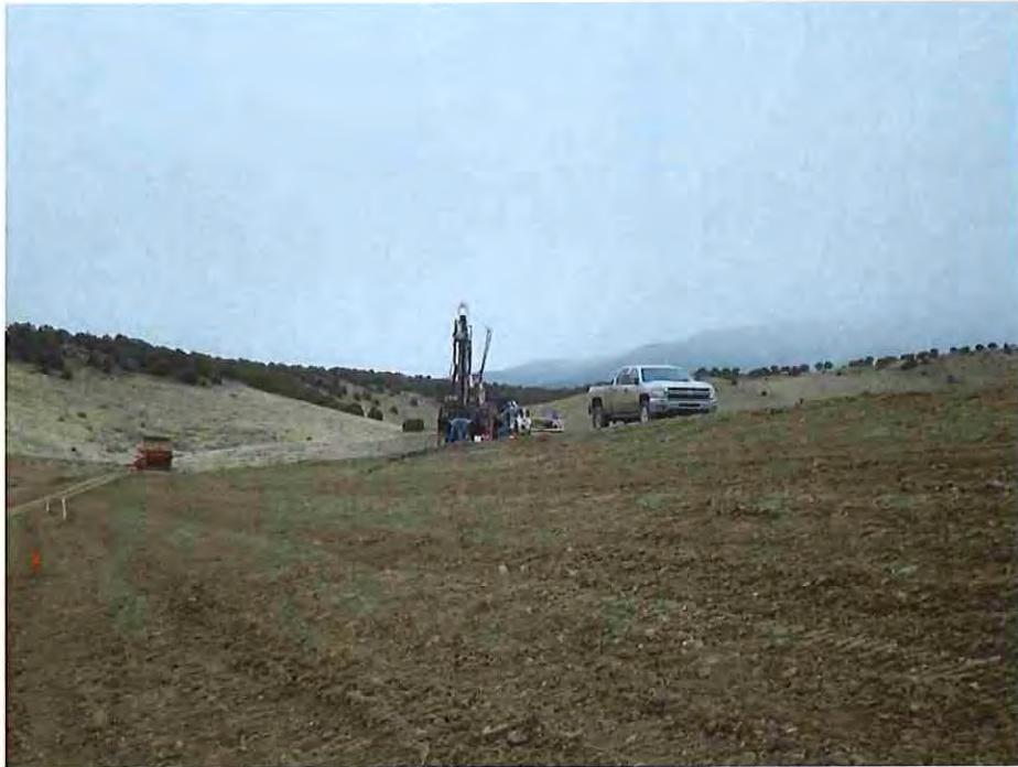
Photo #35: November 28, 2016 – Subcontractor installing the new piezometers along the crest of the dam.
