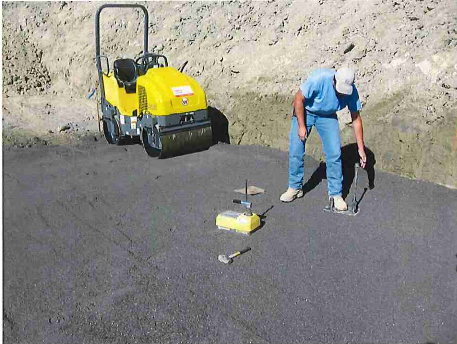
Photo #15: September 27, 2016 – Contractor's quality control subcontractor performing compaction/density tests on the filter sand. A smooth drum roller and the application of clean water was used to compact the filter sand.
