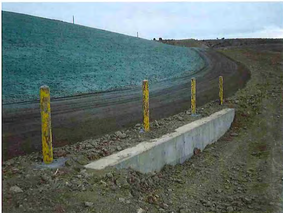
Photo #36: December 15, 2016 – Photo shows the completed retaining wall, pipe bollards, recycled asphalt millings placed on the dam service roads, and seed, fertilizer, mulching operations. Photo is looking south.
