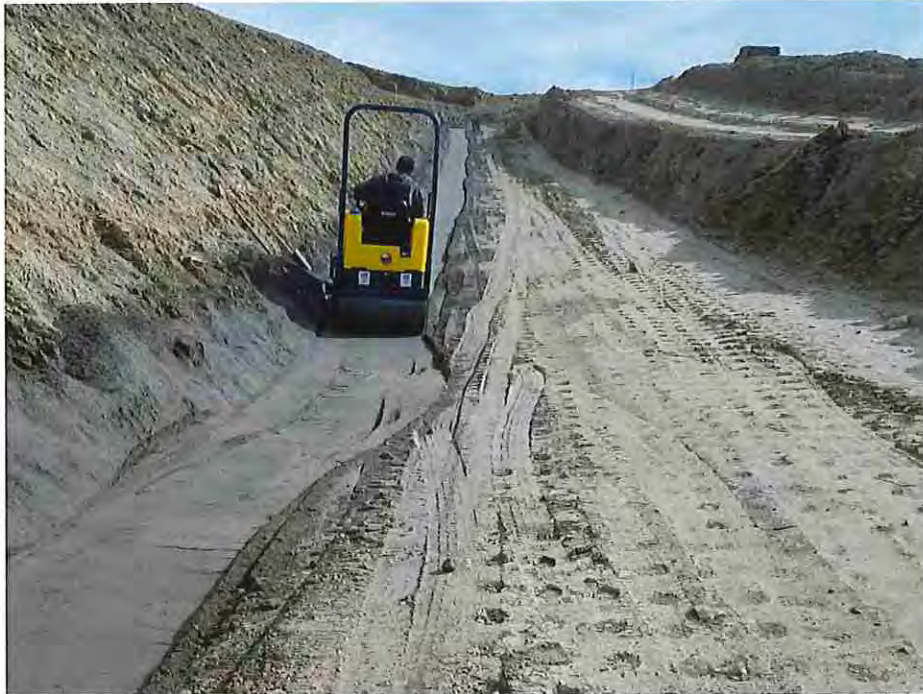
Photo #19: October 3, 2016 – Photos shows the smooth drum roller compacting the filter sand chimney drain, while to the right of the filter sand the embankment fill is being compacted using a large sheep's-foot roller compactor. Indentations from the sheep's-foot roller can be seen in the embankment fill.
