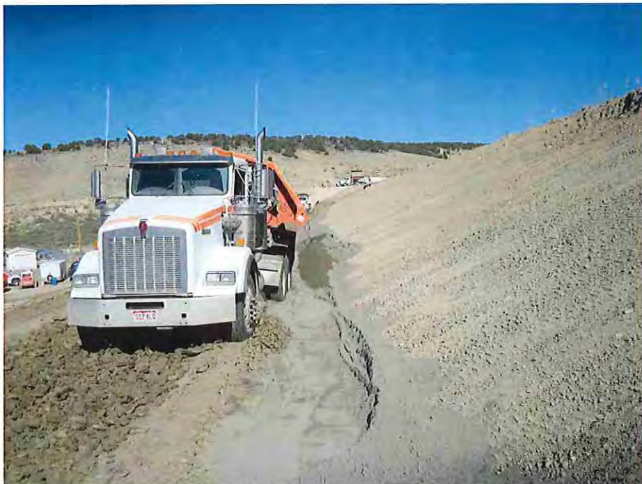
Photo #28: October 21, 2016 – Photo shows contractor's method for placing the filter sand. Side dump trailers were used to place the filter sand. The contractor then used a grader to level the filter sand and then the smooth drum roller compactor would compact the filter sand. A water truck was used to keep the sand wet.
