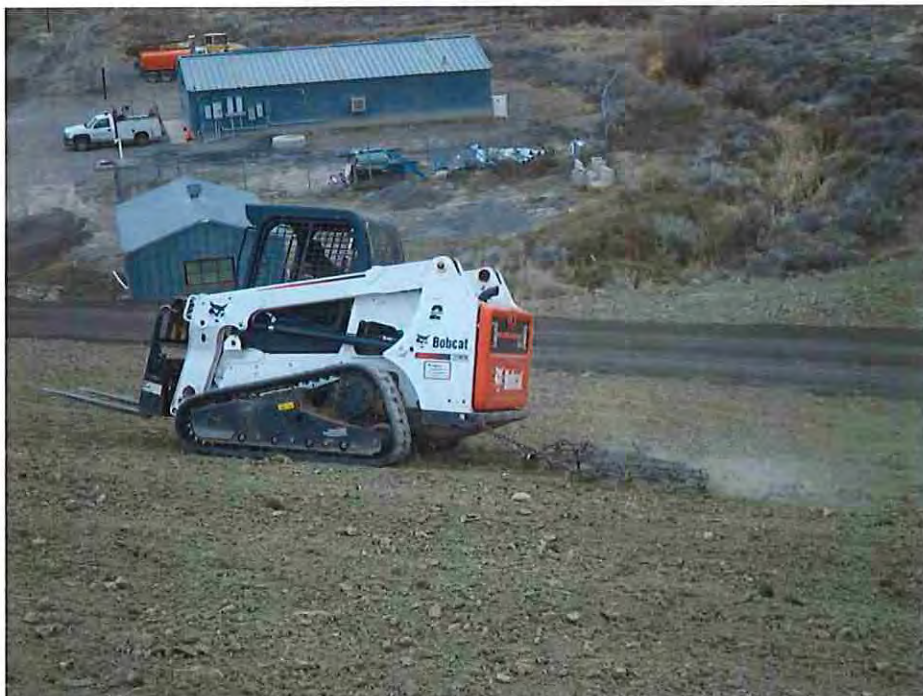
Photo #38: December 15, 2016 – Subcontractor raking the downstream dam face prior to broadcasting native seed, fertilizing and applying mulching.
