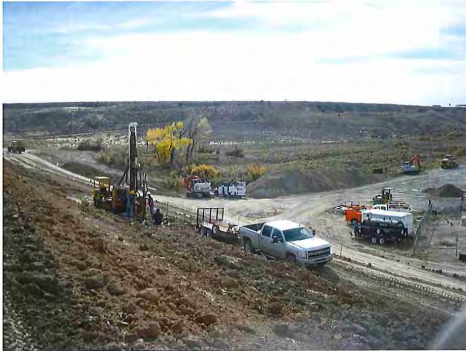
Photo #31: October 28, 2016 – Subcontractor installing the new piezometers along the downstream face of the dam.
