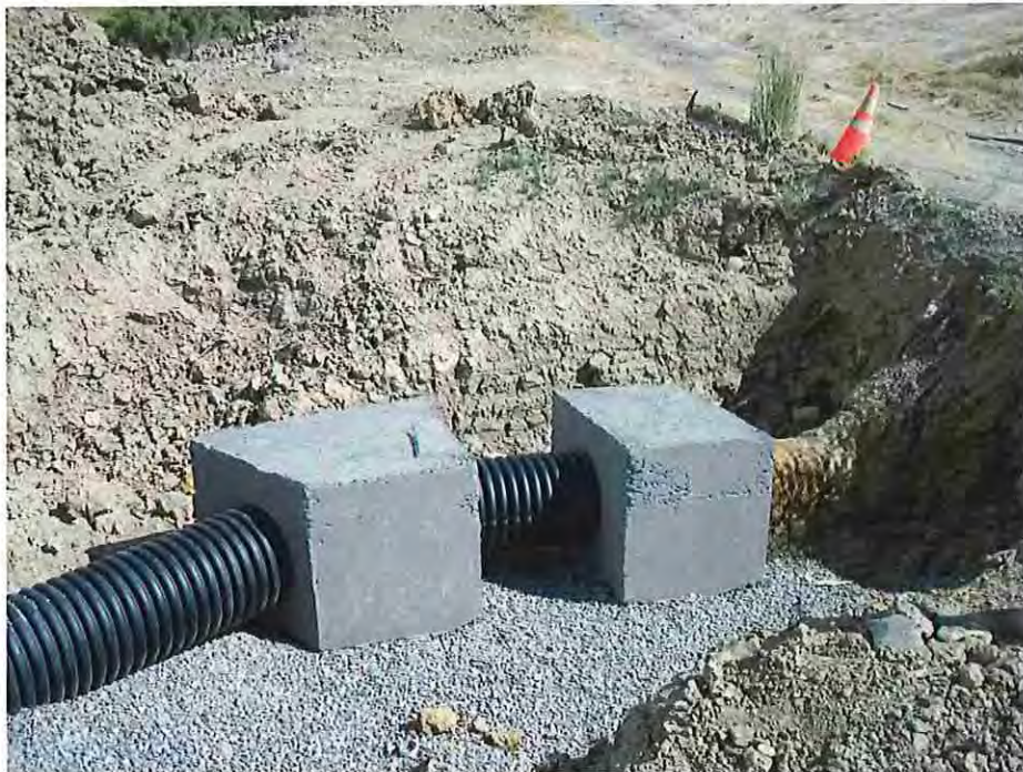
Photo #2: August 17, 2016 – Thrust-blocks poured and backfill operations ready to start. New HDPE pipe was bedded in \frac{3}{4} " minus pipe bedding rock. Backfill material came from the borrow site within the reservoir pool area. Walk behind sheeps-foot roller was used to compact backfill material. Work completed by the City of Grand Junction.
