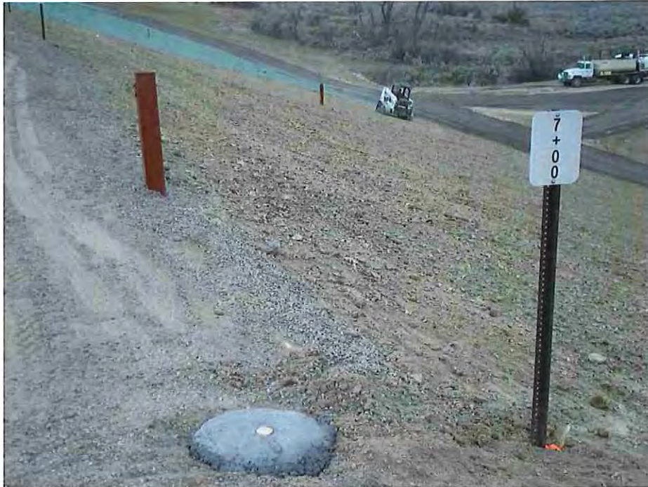
Photo #37: December 15, 2016 – Photo shows the installed piezometers, dam crest station markers, movement monuments set in concrete, and the seeding, fertilizing, mulching operations.
