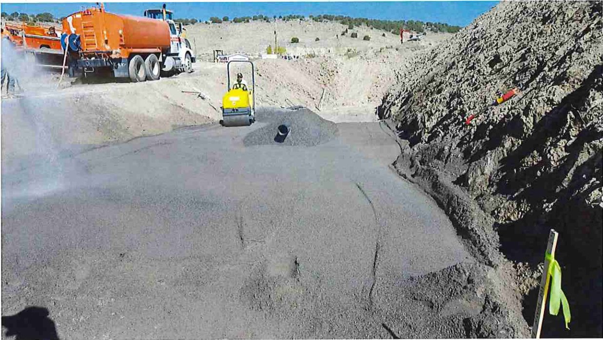
Photo #17: September 27, 2016 – Photo shows the contractor's operations for installing the toe-drain. Water is being applied to the filter sand to keep it wet while the smooth drum roller compacts the sand. Drain gravel is surrounding the pipe.
