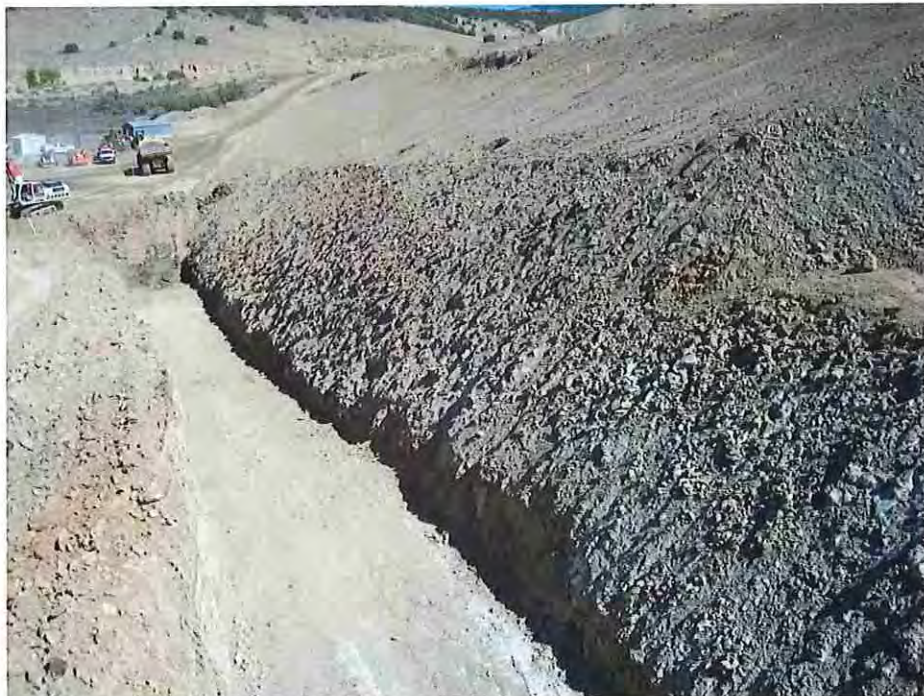
Photo #8: September 15, 2016 – Photo showing the south toe-drain excavation looking north along the dam face.
