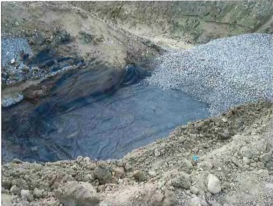
Photo #13: September 22, 2016 – Concrete retaining wall excavation. Soft subgrade conditions existed here as well. Photo shows a separation fabric placed directly on the soft subgrade with geogrid and stabilization rock placed on top. As-built detail of retaining wall subgrade shown within the As-Built set of construction plans.
