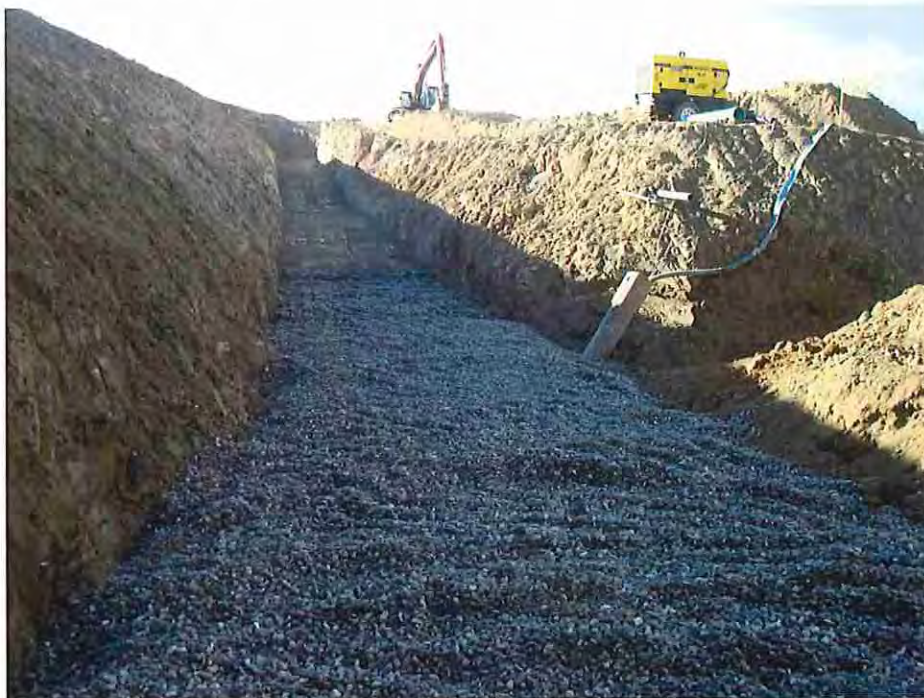
Photo #12: September 22, 2016 – Photo showing completion of the rock stabilization zone with the contractor's bypass pumping equipment set up. Filter sand would be placed on top of this stabilization rock.
