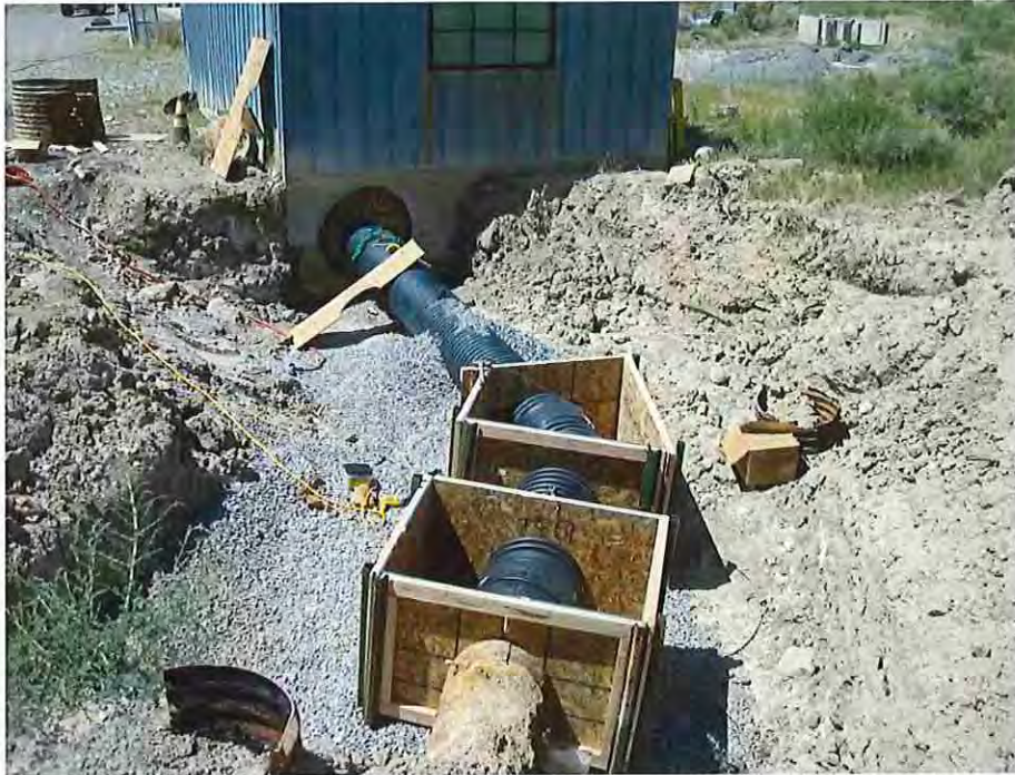
Photo #1: August 10, 2016 – Installation of new 18" dia. HDPE Corrugated pipe for the reservoirs low-level outlet pipe. The wood form boards are for the concrete thrust-blocks. Work completed by the City of Grand Junction.
