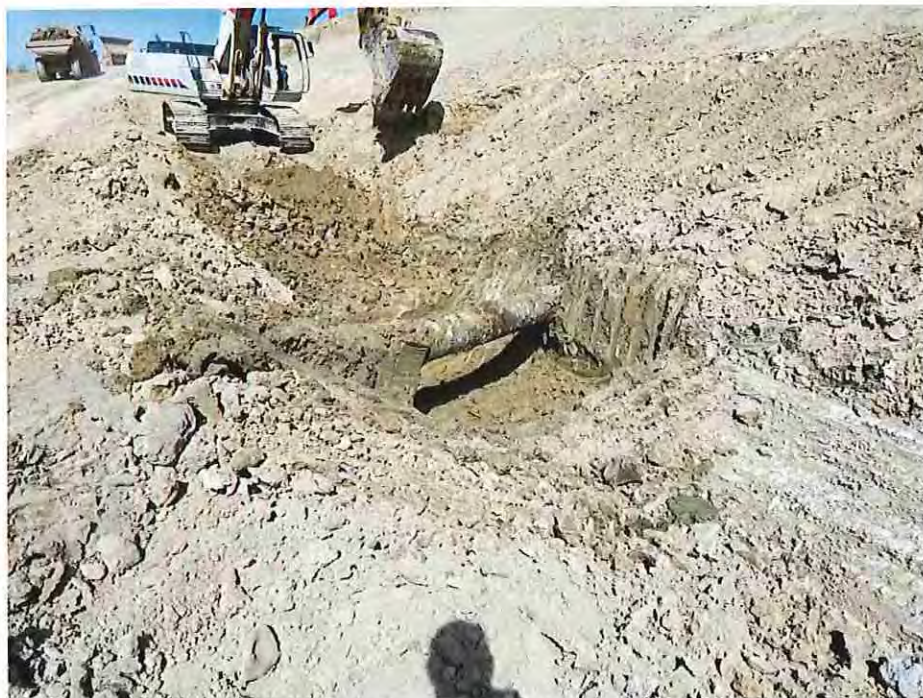
Photo #20: October 5, 2016 – Excavation of the north toe-drain. This photo shows the contractor excavating around the reservoir's low-level outlet pipe. The toe-drain would be installed underneath the low-level outlet pipe. Installation details are shown in the As-Built construction plans.
