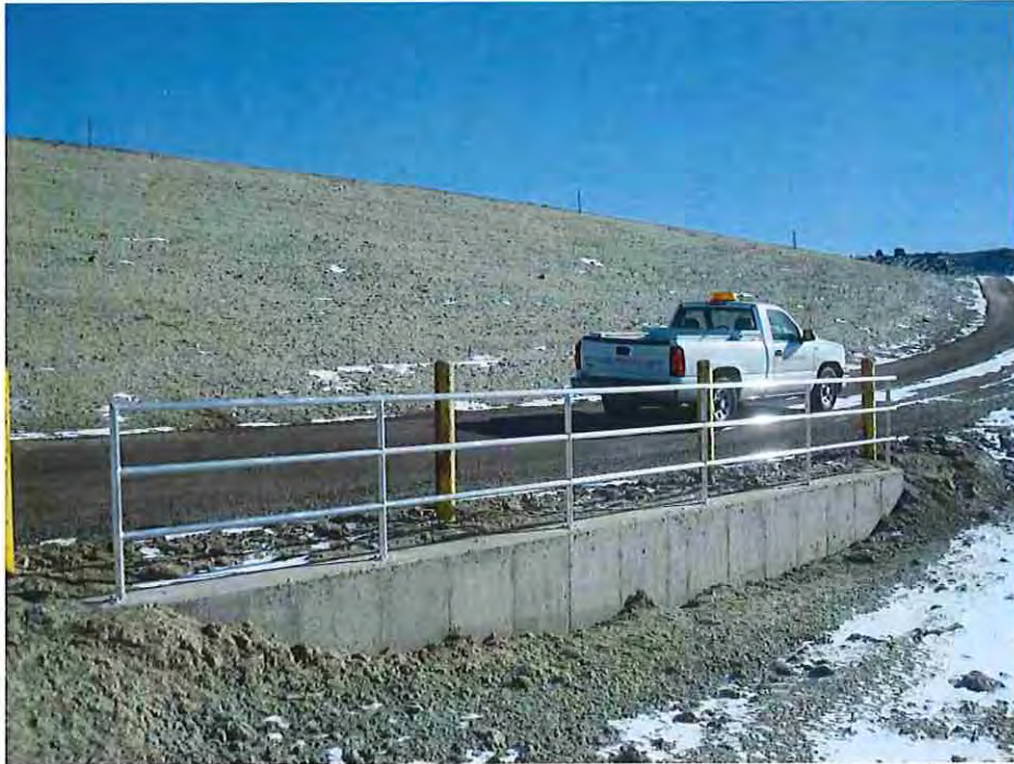
Photo #39: December 27, 2016 – Aluminum hand railing installed along the top of the retaining wall.
