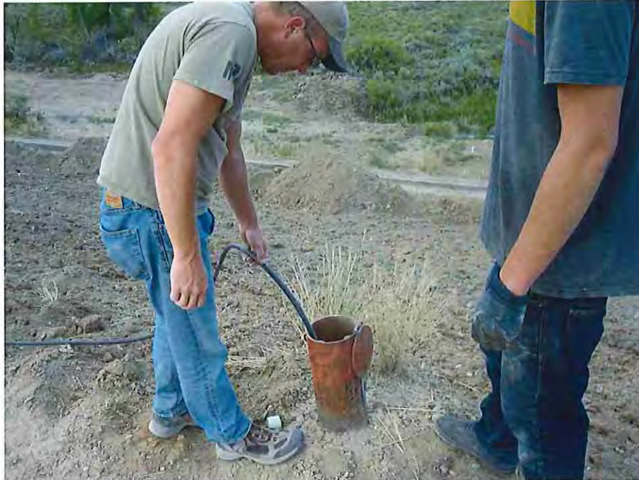
Photo #3: September 3, 2016 – Subcontractor, Huddleston-Berry Engineering, abandoning the dams old piezometers using a cement-bentonite grout.
