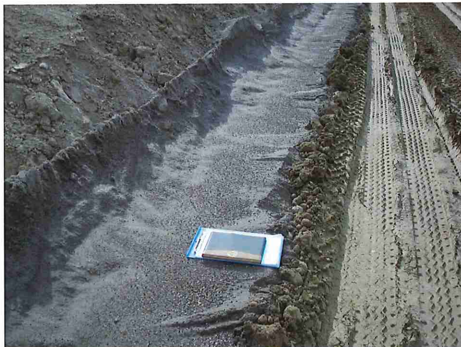
Photo #22: October 17, 2016 – Photo showing the 3-ft wide filter sand chimney and the embankment fill to the right.
