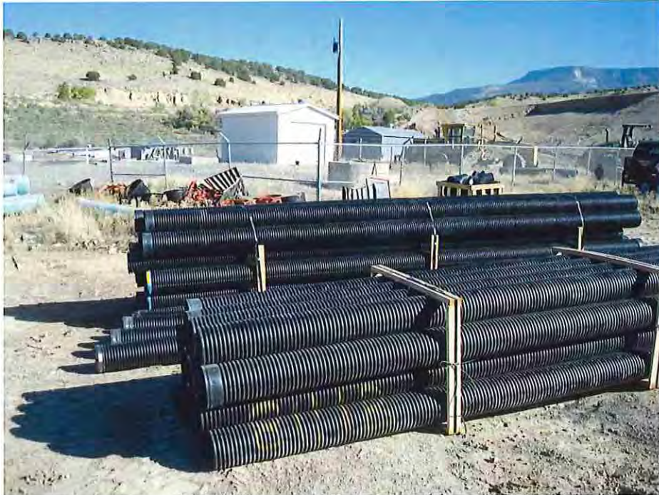
Photo #7: September 15, 2016 – The 8" dia. HDPE perforated toe-drain pipe is delivered and stockpiled on-site.
