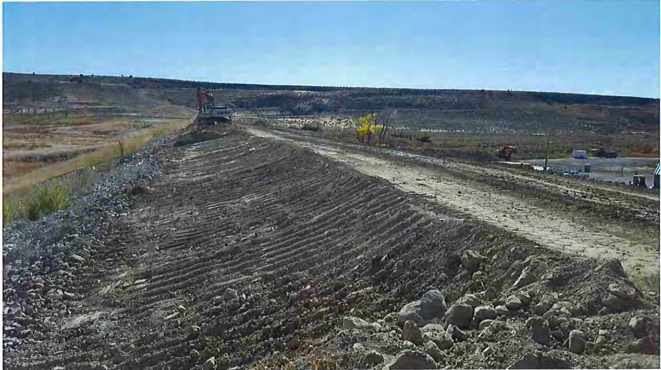
Photo #32: November 2, 2016 – Contractor stripping and prepping the upstream face of the dam crest for the placement of drain gravel and riprap.
