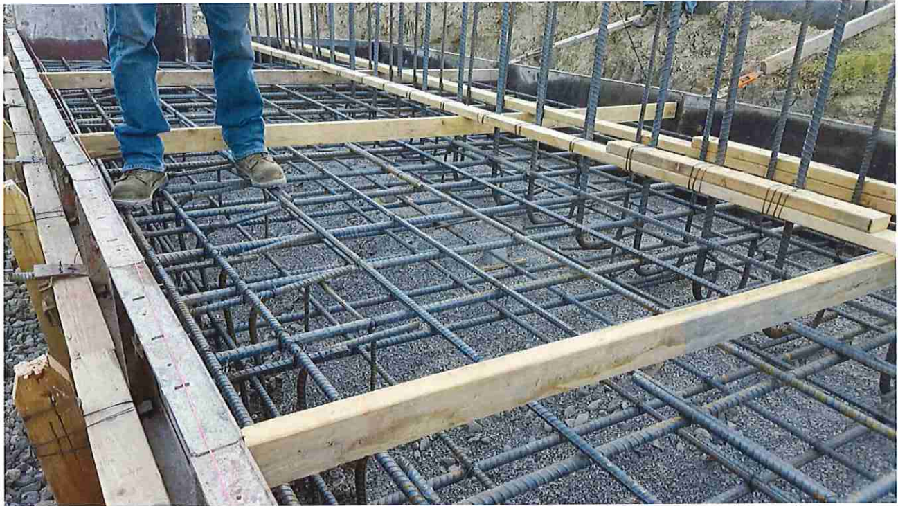
Photo #21: October 10, 2016 – Steel reinforcement for the footer of the concrete retaining wall.
