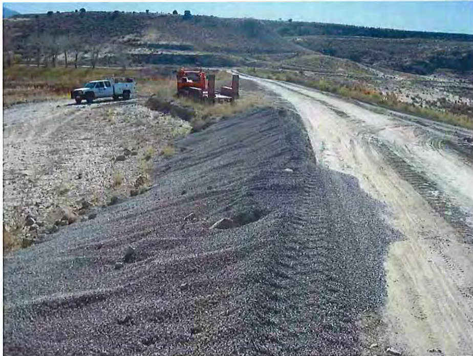
Photo #33: November 15, 2016 – Drain gravel placement along the upstream face of the dam. Riprap protection will be placed on top of the drain gravel.
