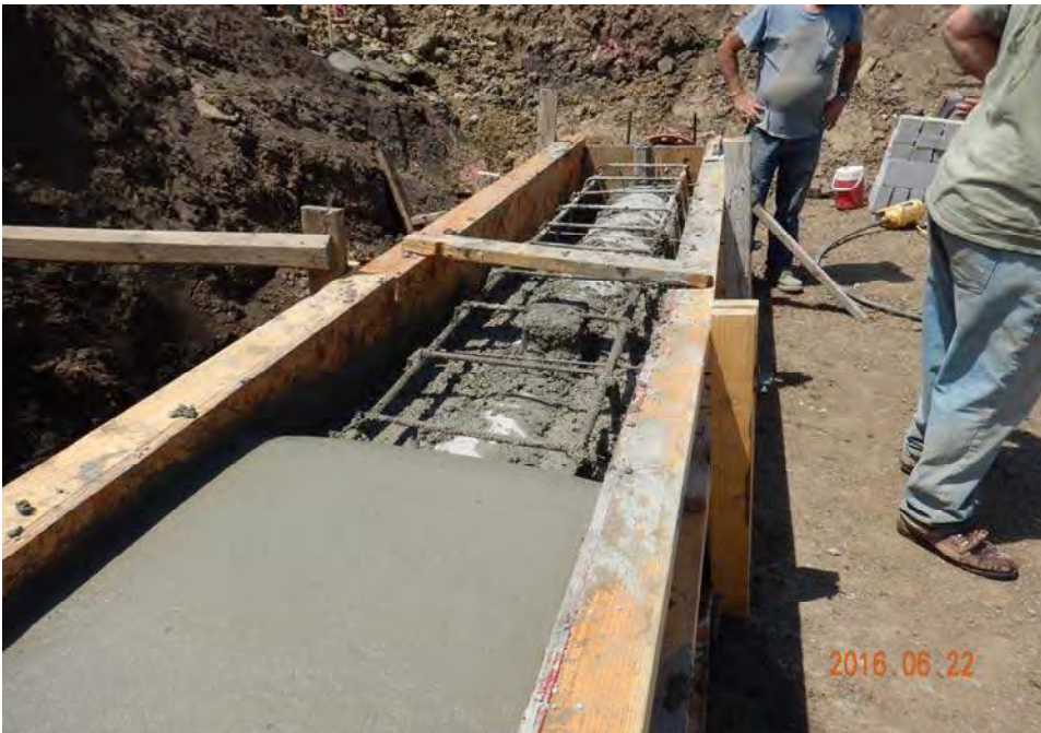
Photograph 28: Portion of the conduit encasement that was not complete with the rest of the encasement (OW Sta. 1+17 to OW Sta. 1+27).
