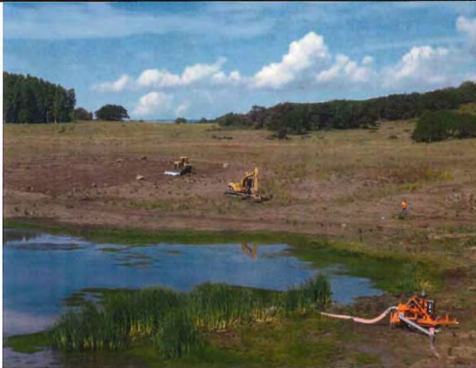
Looking from the dam breach to the borrow area upstream of the dam.
