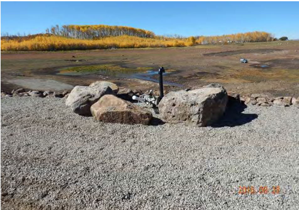
Photograph 40: Boulders placed around the hand wheel pedestal for protection.
