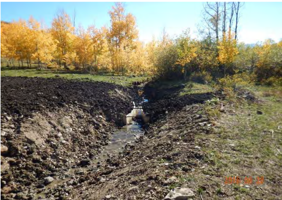
Photograph 42: Parshall flume in the discharge channel.
