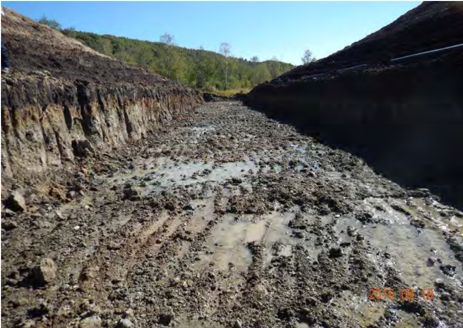
Photograph 3: Bottom of excavation without effective dewatering.
