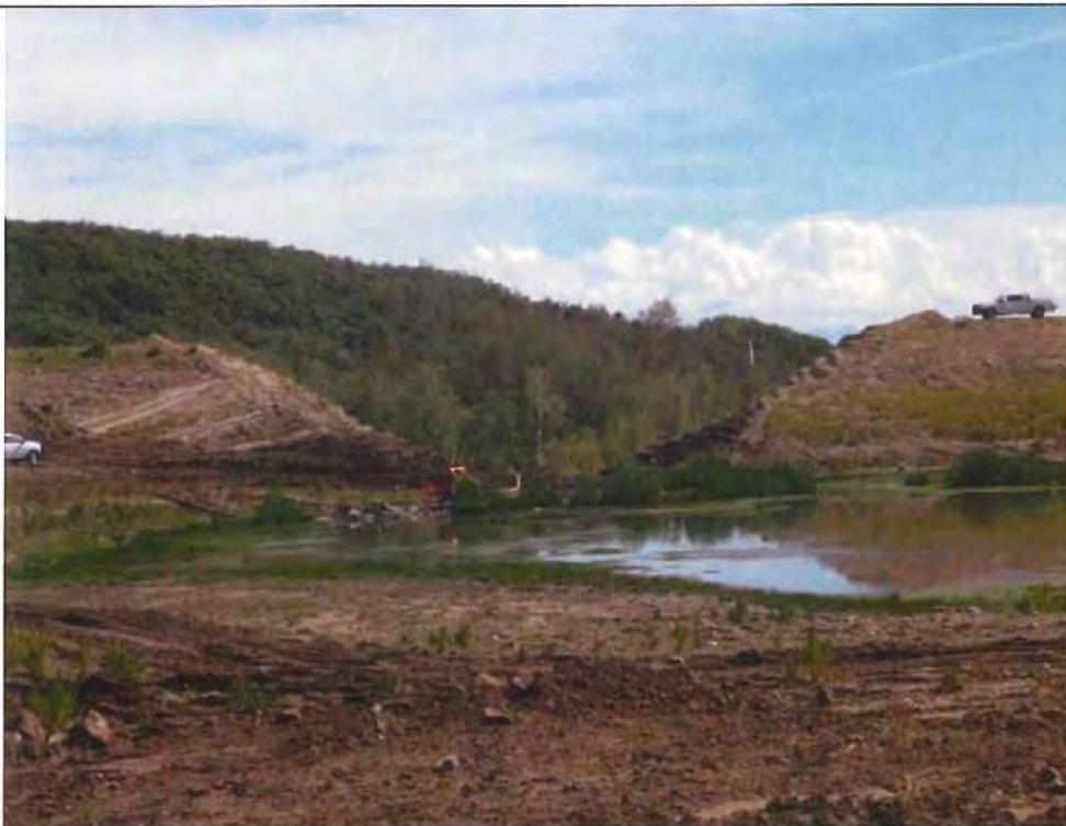
Looking from the borrow area toward the dam breach.
