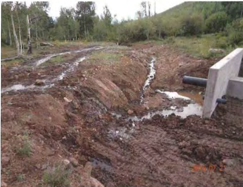
Photo 1 – Water flowing around downstream headwall.
