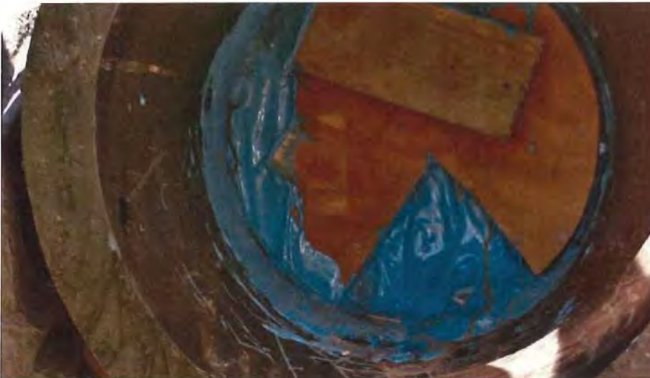
Photo 1 – End plug for the outlet works conduit (HDPE pipe).
