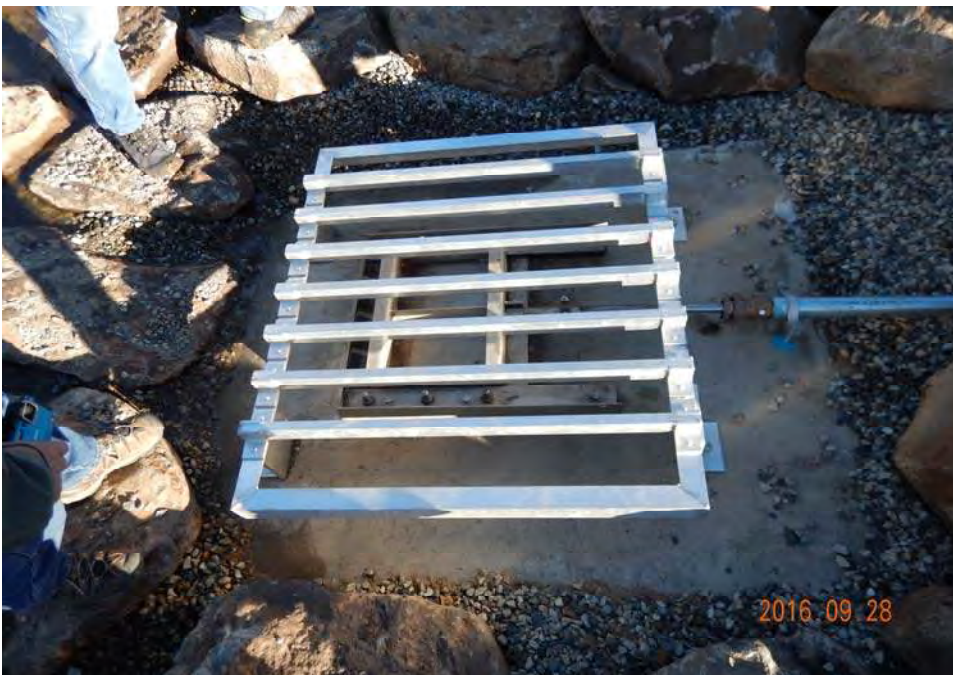
Photograph 38: Inlet trash rack and gate.
