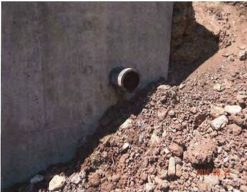
Photo 3 – Flow from the sand collar drain pipe.
