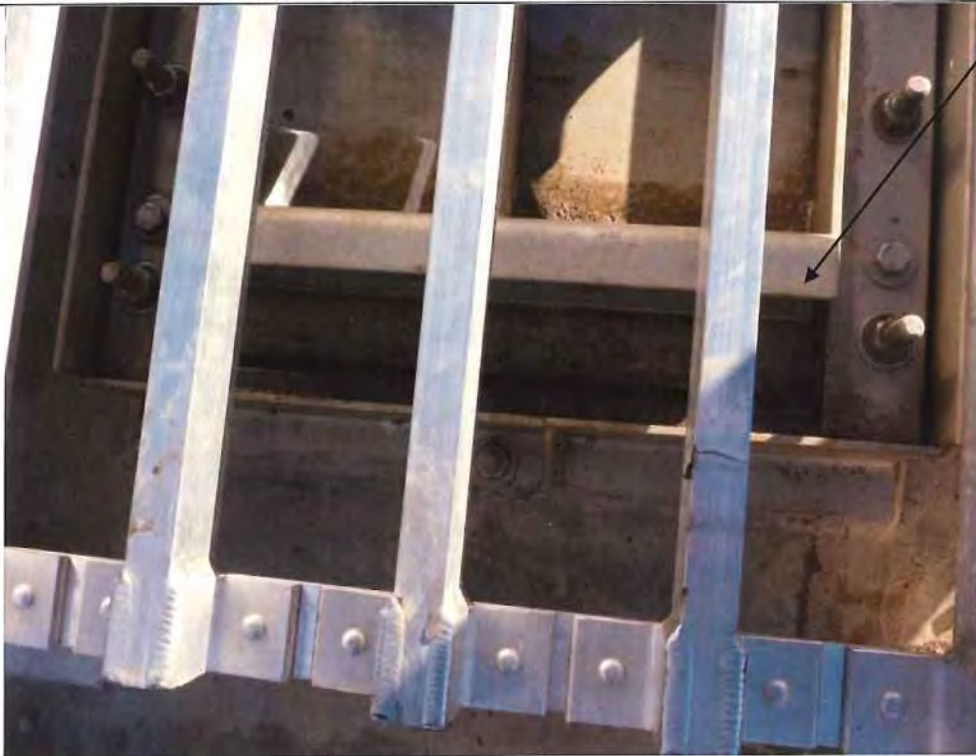
Right corner (looking downstream) of gate closes barely sooner than left side, gate appears to seal adequately.
