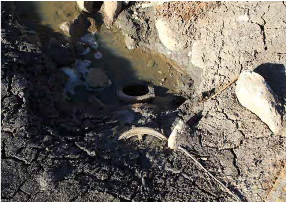
Photograph 24: Existing valve on upstream end (outlet works inlet).
