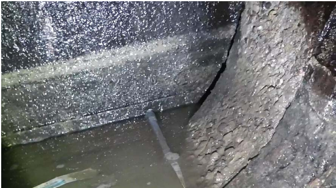
Screenshot 12: View looking upstream at control gate in Conduit No. 2. Note significant scour to pipe immediately downstream of control gate. November 9, 2016.
