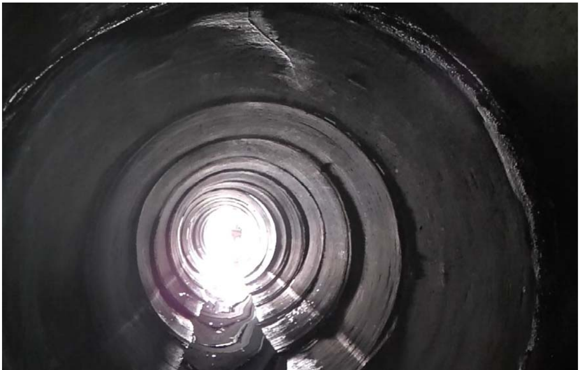
Screenshot 8: View looking downstream in Conduit No. 2 at Station 0+39 feet downstream of gate. View shows cracking in the pipe crown, disjointedness, and movement of pipe sections. November 9, 2016.
