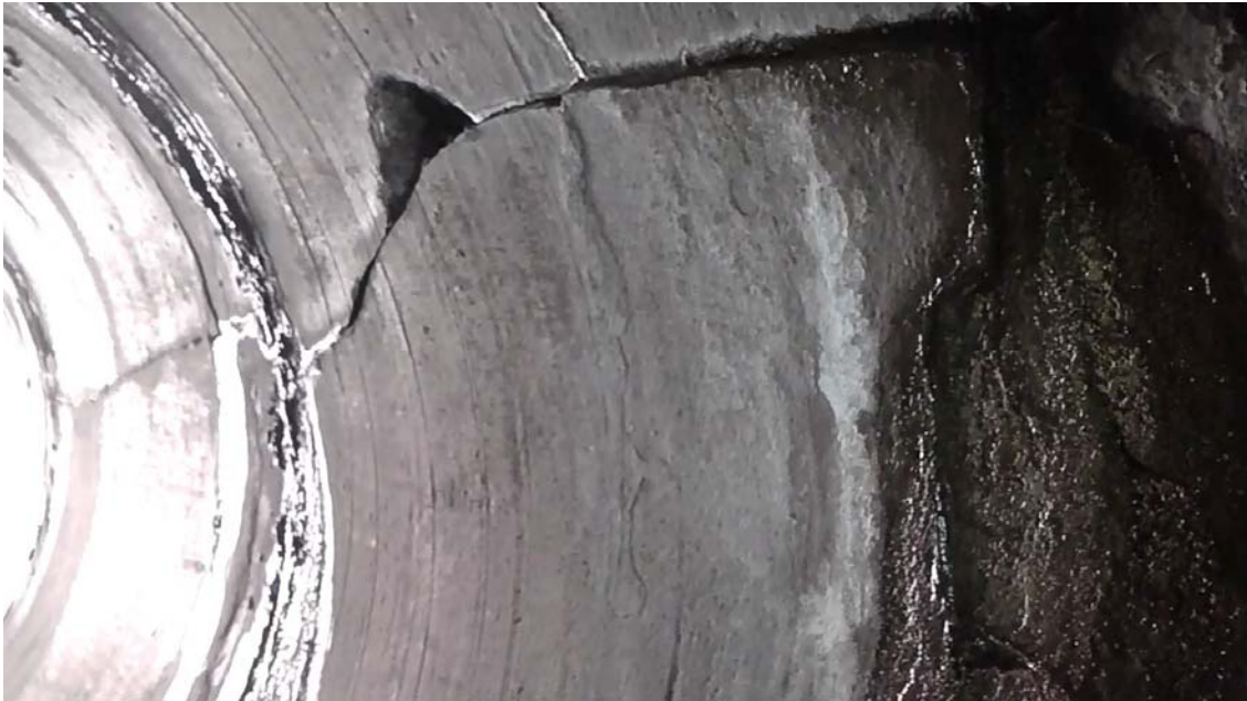
Screenshot 3: View of circumferential crack with seepage and longitudinal crack running length of pipe, in Conduit No. 2 at Station 0+82 feet downstream of gate, looking downstream. Note piece of pipe missing above longitudinal crack. November 9, 2016.
