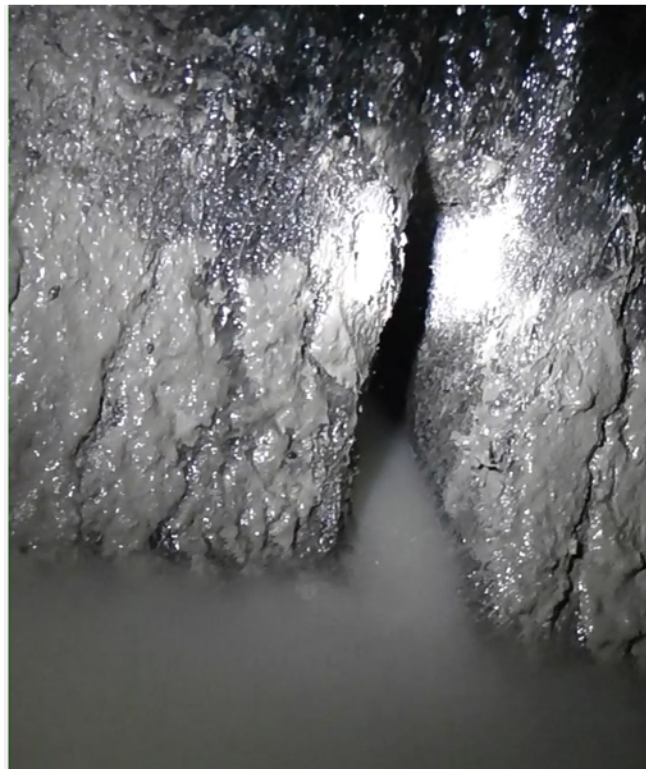
Screenshot 6: Gap in previously repaired pipe joint at bottom. Located in Conduit 4 at Station 0+81 feet downstream of gate. November 9, 2016.
