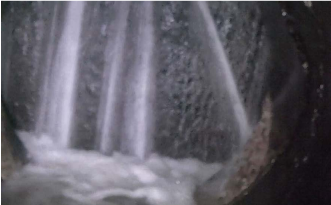
Screenshot 11: View looking upstream at control gate in Conduit No. 3. Note significant leakage around control gate and scour to bottom and sides of pipe. November 9, 2016.
