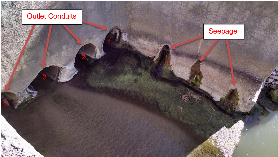
Photo 2: View of the outlet works terminal structure and outlet conduit outfalls from the right wing wall, looking upstream. Note seepage from the weep holes in the left wing wall and gate leakage and seepage flows exiting from the outlet works conduits. November 9, 2016.
