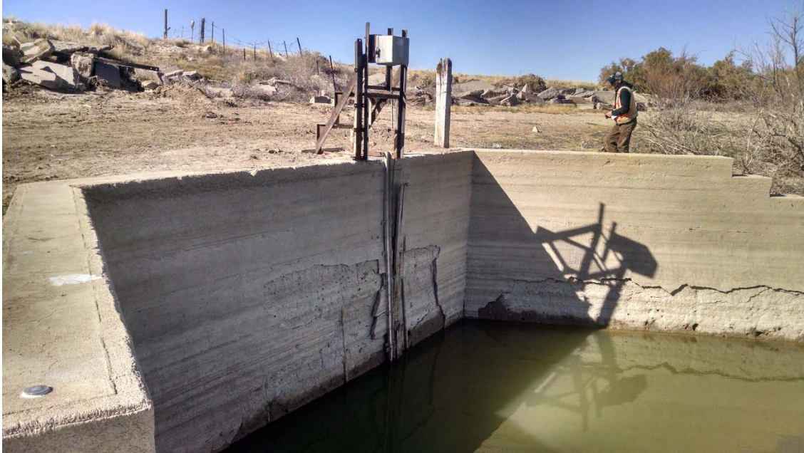
Photo 1: View of the outlet works intake structure from the left wing wall, looking downstream towards the dam. The reservoir elevation was 19.40 feet on the staff gauge on date of inspection. Note the concrete deterioration. November 9, 2016.
