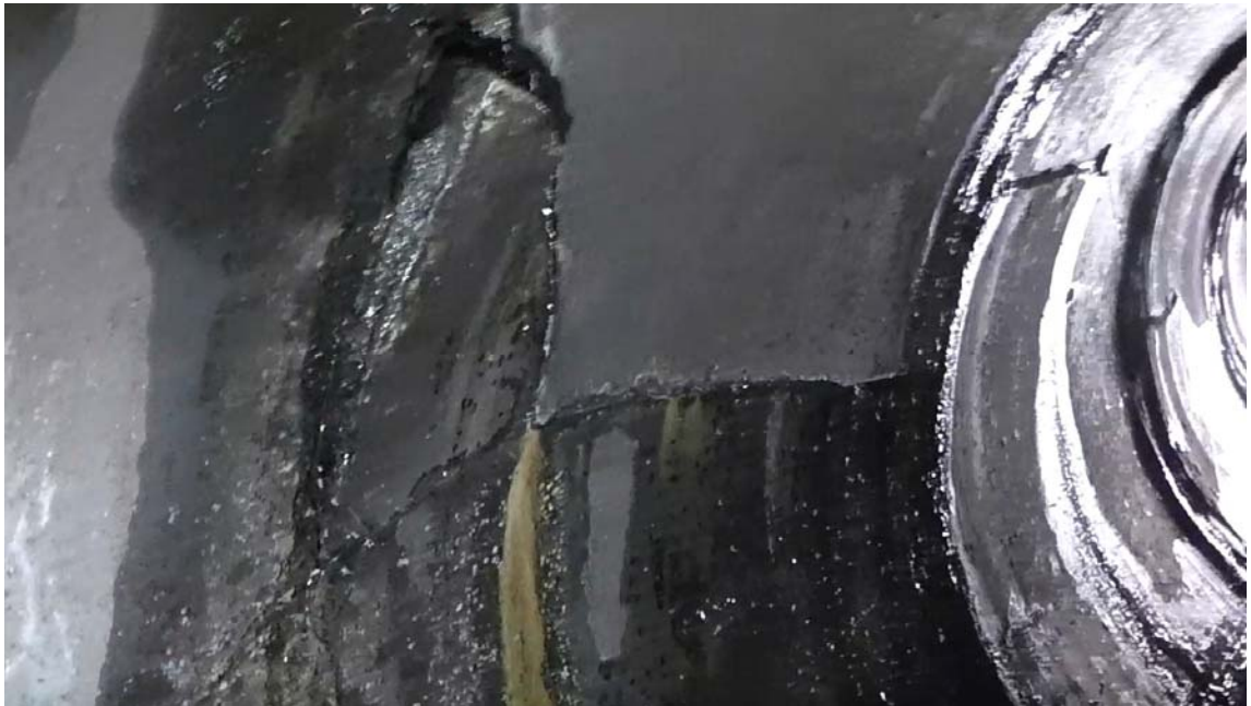
Screenshot 5: View looking downstream in Conduit No. 3 at Station 0+81 feet downstream of gate. Note cracking and movement of a piece of the pipe wall. November 9, 2016.
