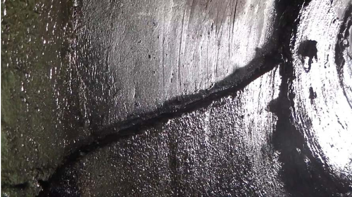
Screenshot 1: View of longitudinal crack running length of pipe section with 1/4" lateral displacement, in Conduit No. 1 Station 0+89 feet downstream of gate, looking downstream. November 9, 2016.
