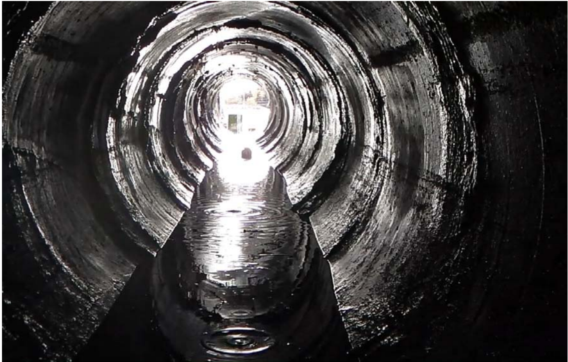
Screenshot 7: View looking downstream in Conduit No. 1 at Station 0+69 feet downstream of gate. Significant seepage, disjointedness and cracking in the pipe was observed from this point to the conduit discharge end. November 9, 2016.
