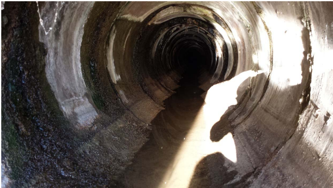
Photo 8: View of Conduit No. 4 taken from the discharge end looking upstream. Note lateral offset of joints and seepage from joints and cracks in pipe. November 9, 2016.
