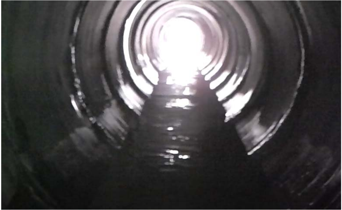
Screenshot 9: View looking downstream in Conduit No. 4 at Station 0+23 feet downstream of gate. View shows disjointedness and movement of pipe sections. November 9, 2016.
