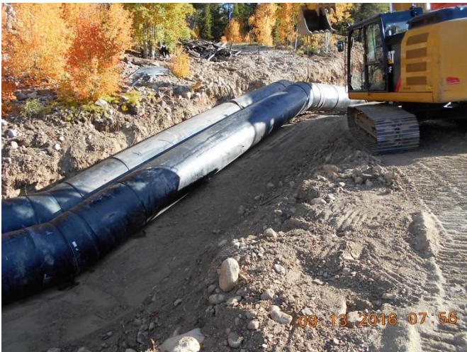
48" HDPE Elbows Upstream of Outlet
