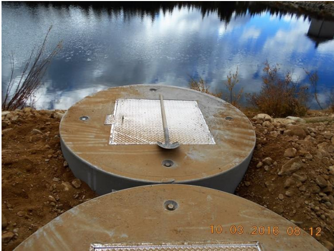
Hatches Over Access Manways
