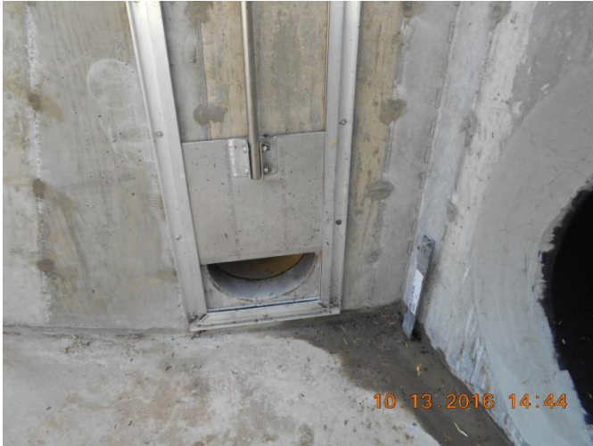
Reservoir Intake Slide Gate
