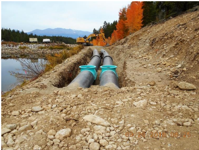
Manway Access Hatches in Pipeline
