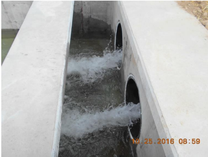
Steam Water Exiting Pipes at Outlet Structure
