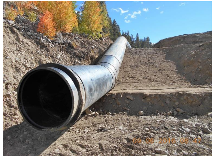
48" HDPE at Discharge
