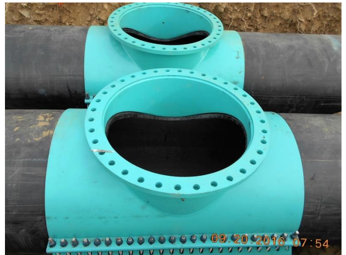
Close-up of Manway Hatches
