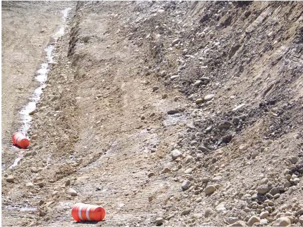
Water along toe of western berm area.
