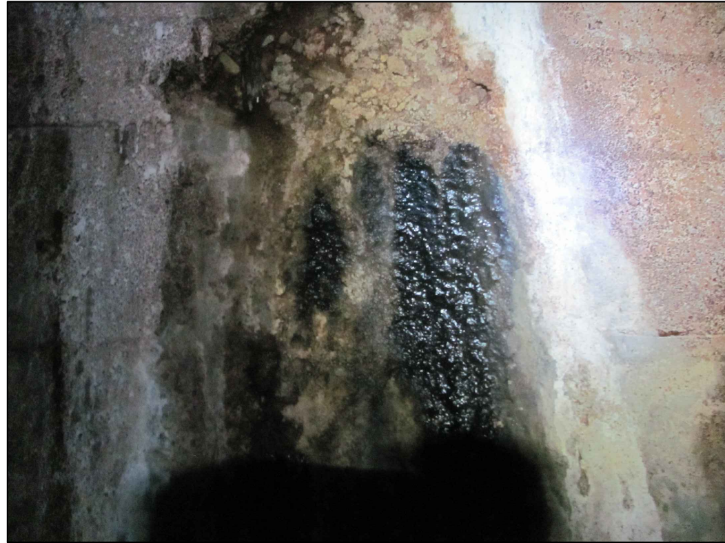
LEAKS TO BE SEALED
