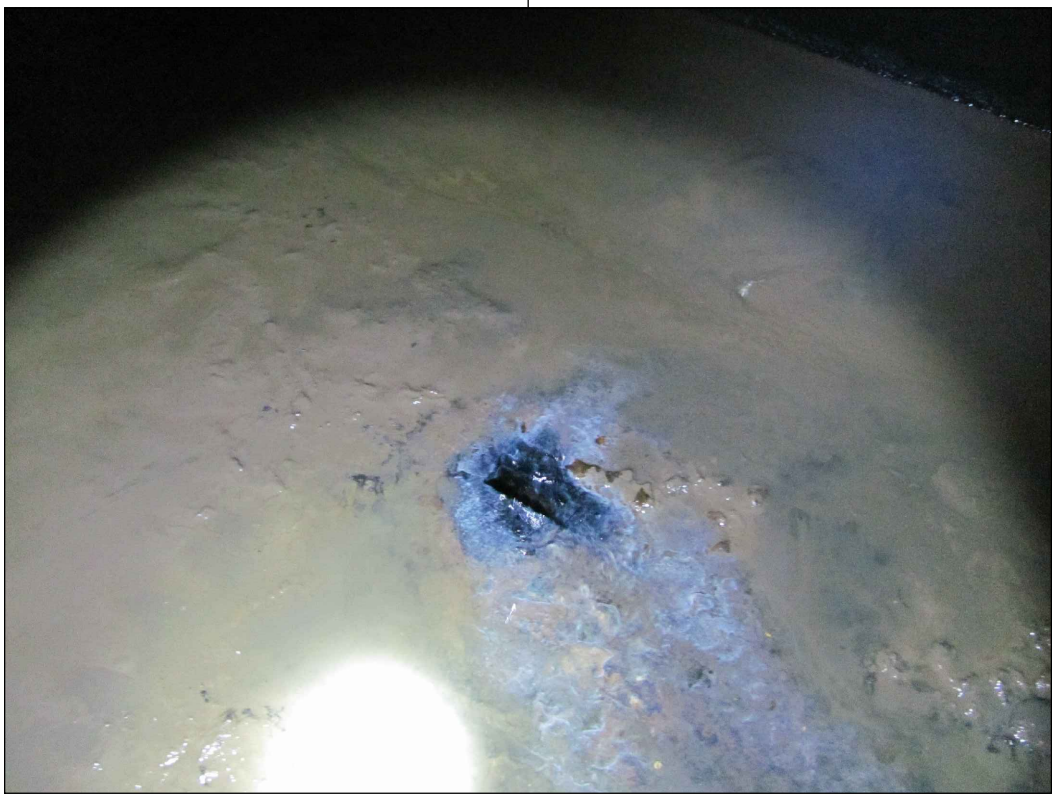
HOLE/LEAK IN FLOOR SLAB
