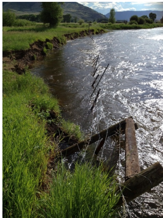
Figure 1-6. Severe Bank Erosion on Reeder Creek Ranch.
