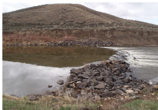
Figure 1-3. Diversion Drop Structure installed by Northern Colorado Water Conservancy District in 2004.
