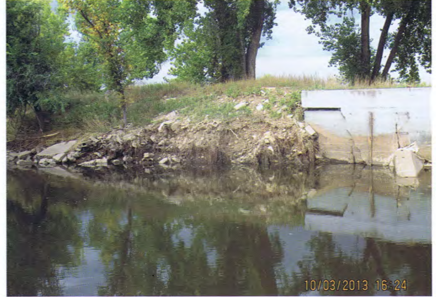
Fossil Creek Reservoir Inlet Ditch left bank abutment
