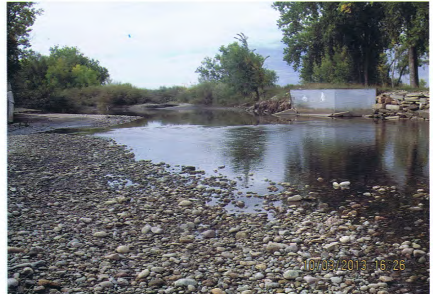
Fossil Creek Reservoir Inlet structure destroyed
