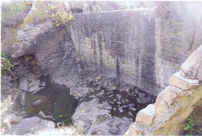
Drop structure below the Cheyenne Diversion above Clark Lake . . . a must repair project
