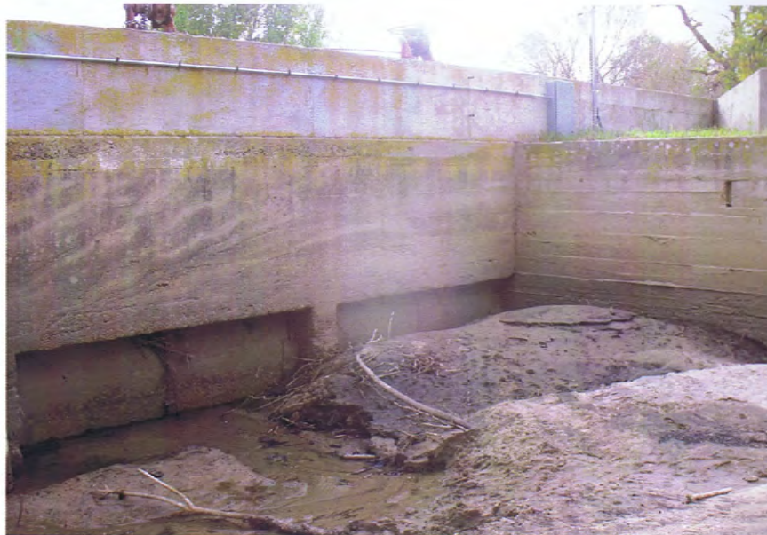
Silt Deposit Radial Gates at FCRID
