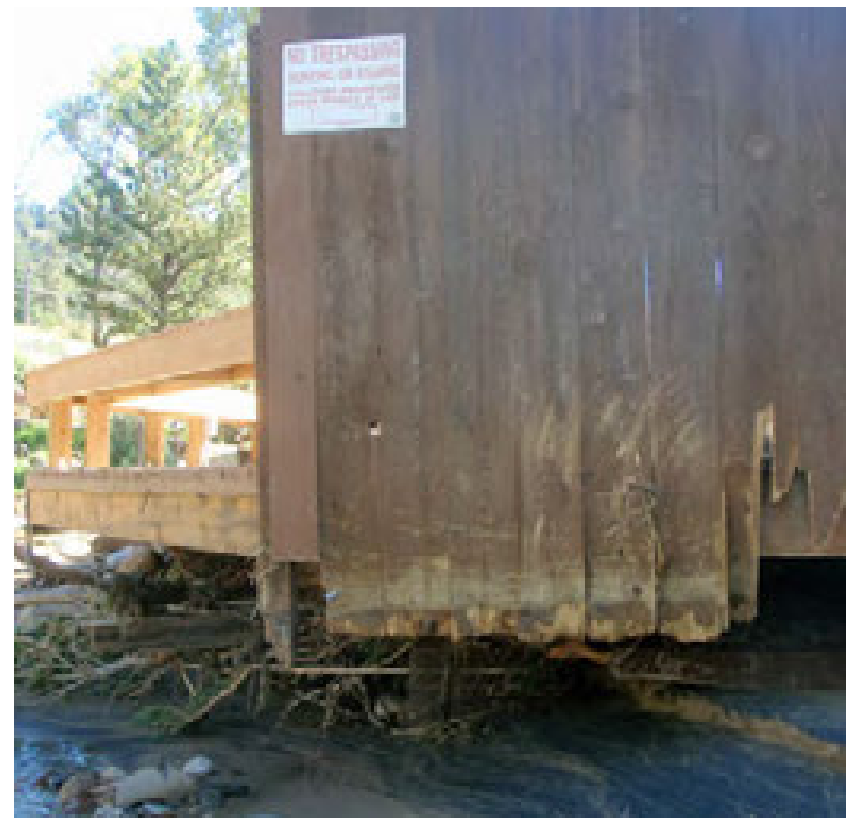
Fall River Structure Damage
