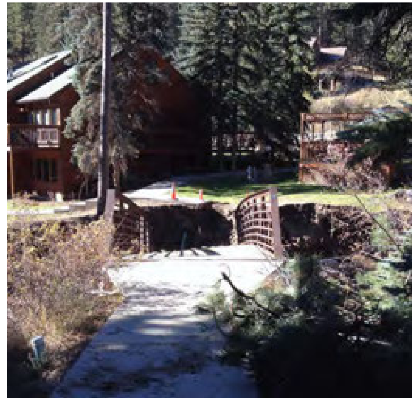
Fall River Pedestrian Bridge Damage
