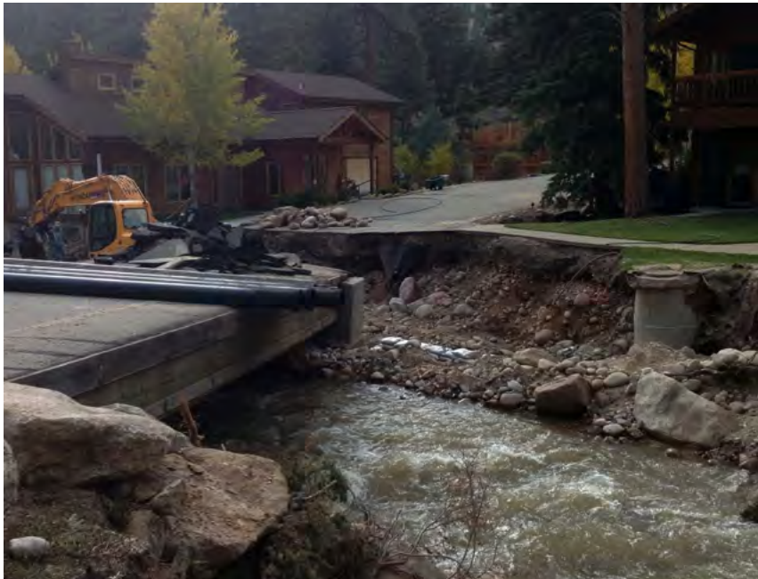
Bridge and Utility Damage
