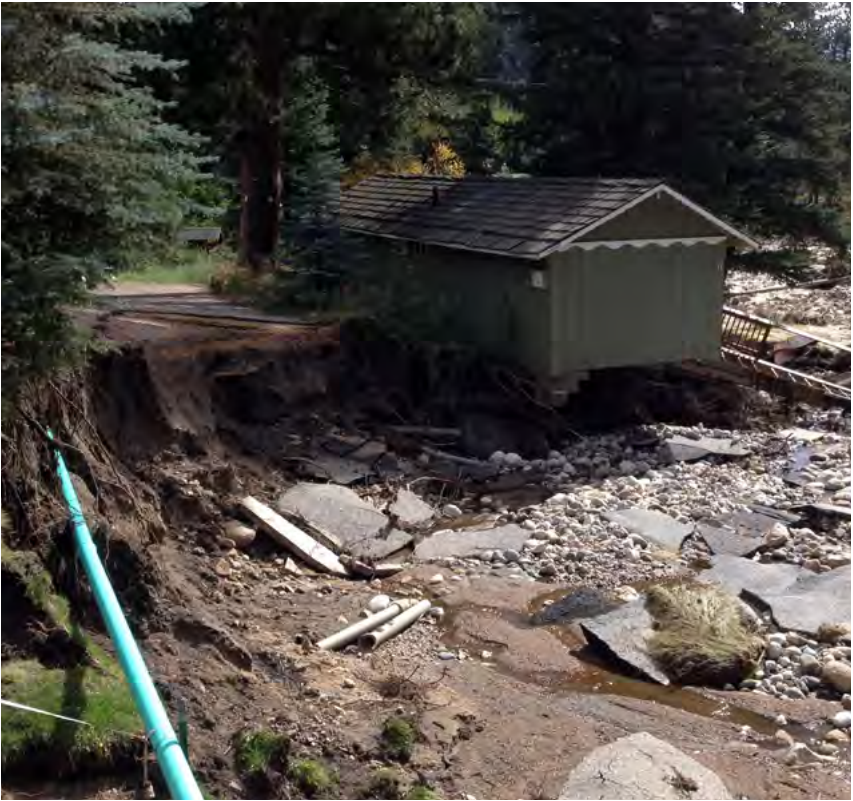
Utility and Structure Damage
