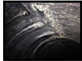
HOLES IN TUNNEL PIPE
