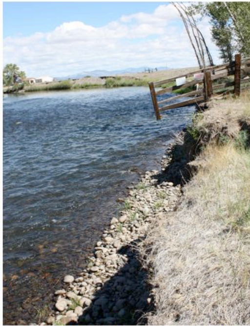
Figure 12. Example of Steep, Eroding Streambanks in the Project Area
