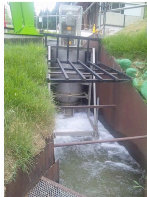
Figure 23. Typical Micro-hydro Power Production Facility
