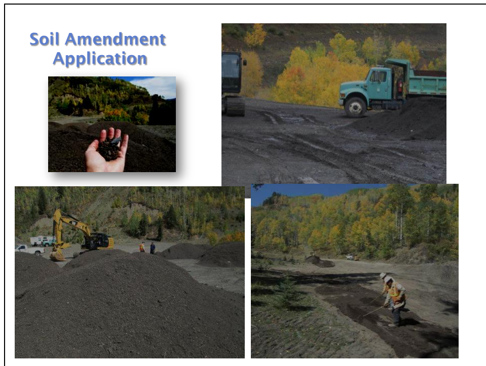
Figure 14. Application of biochar/compost and compost only soil amendments in treatment areas. Top left photo is a close up of biochar. Piles in photos are compost/biochar blend.
