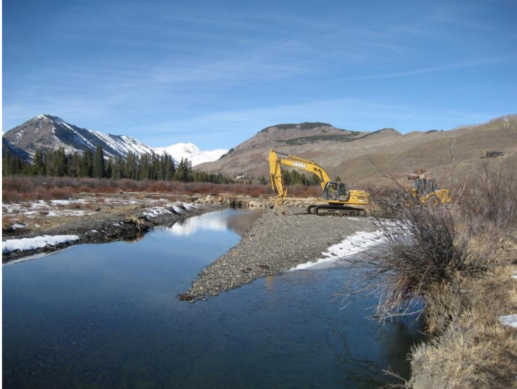
Pre-work gravel bar obstructing natural bend
