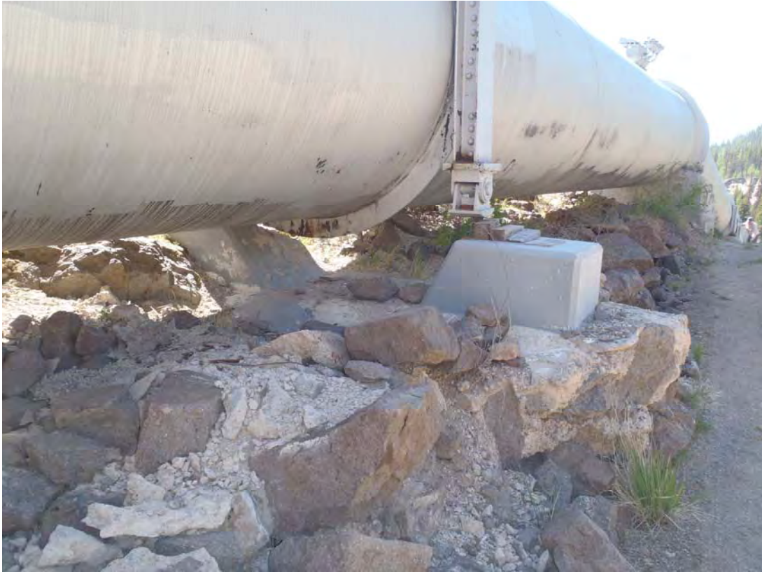
11. Looking downstream along the siphon, just upstream of the second thrust block. Third pier support in foreground. Rocker pad is lifted above pier due to foundation slide area.
