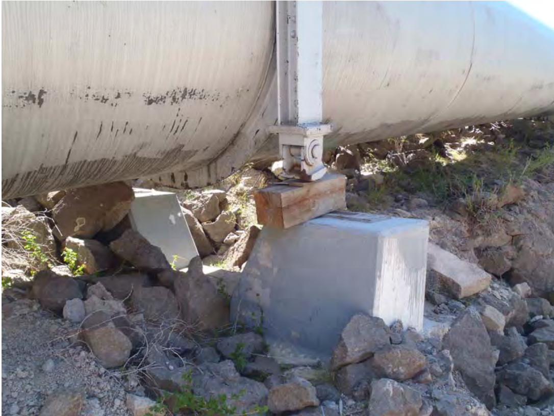
13. Looking downstream along the siphon, just upstream of the second thrust block. Fifth pier support in foreground. Rocker pad is lifted above pier due to foundation slide.
