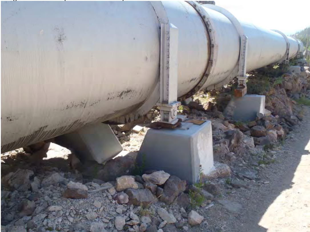
14. Looking downstream along the siphon, just upstream of the second thrust block. Sixth pier support in foreground. Rocker pad is lifted above pier due to foundation slide.
