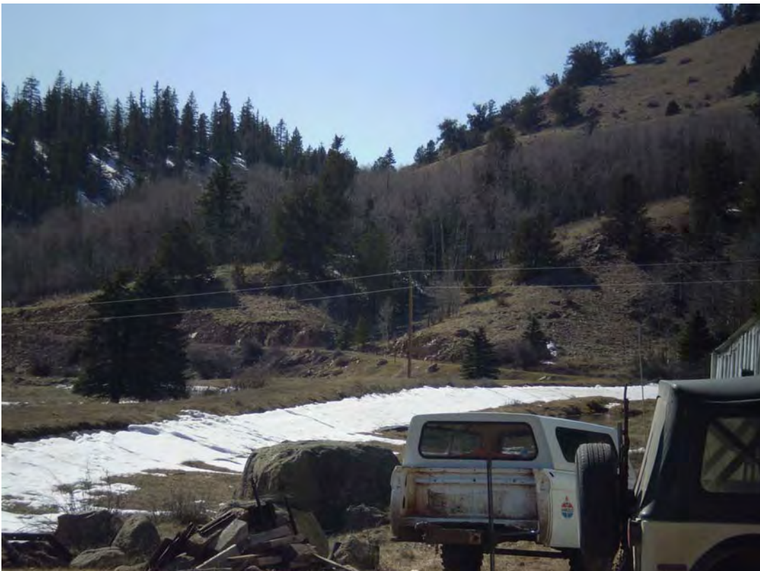
11. Looking upstream along the canal with the slide area in background. The canal was construction on top of the slide area. The canal is seeping along this area.
