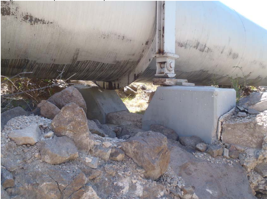
12. Looking downstream along the siphon, just upstream of the second thrust block. Fourth pier support in foreground. Rocker pad is lifted above pier due to foundation slide.
