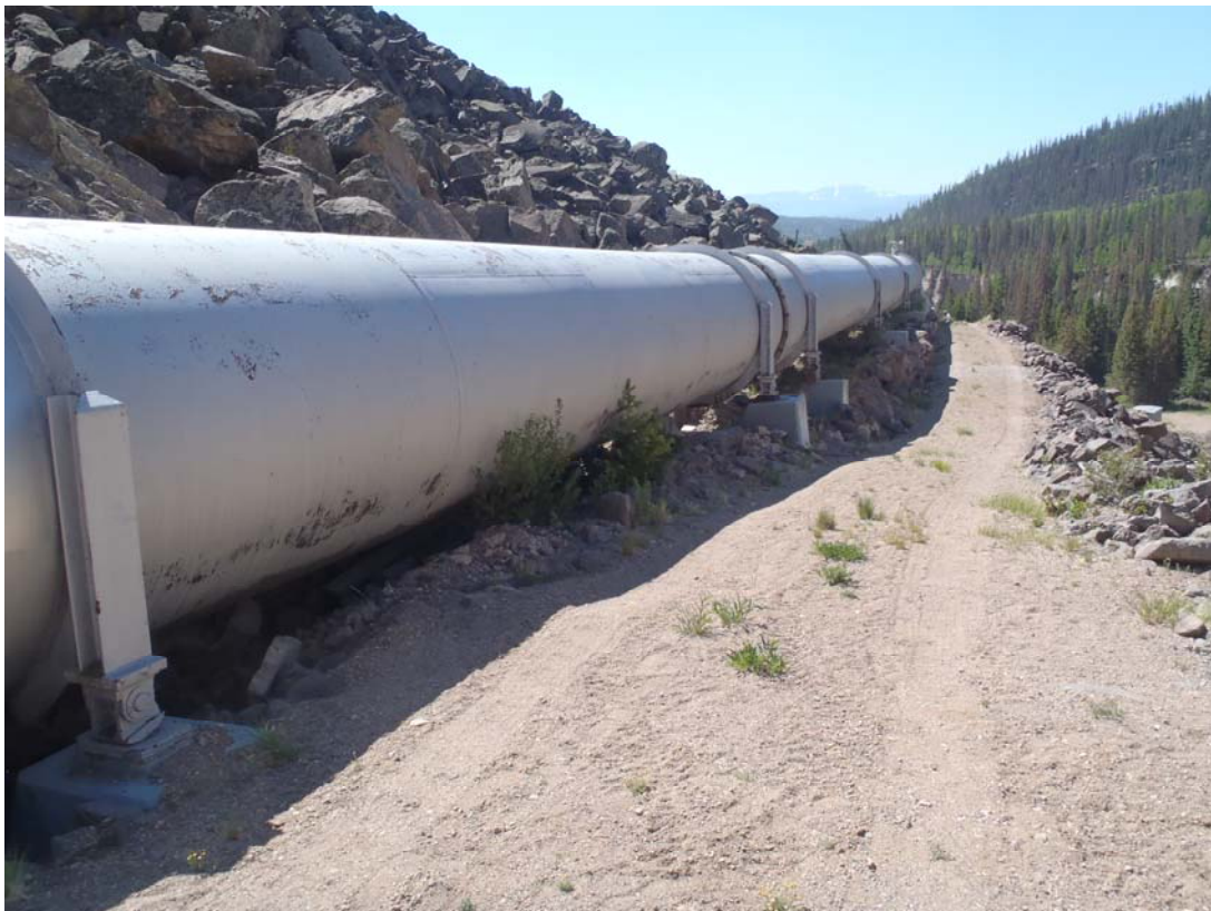
16. Looking downstream along the siphon through the slide area that is impacted the piers.
