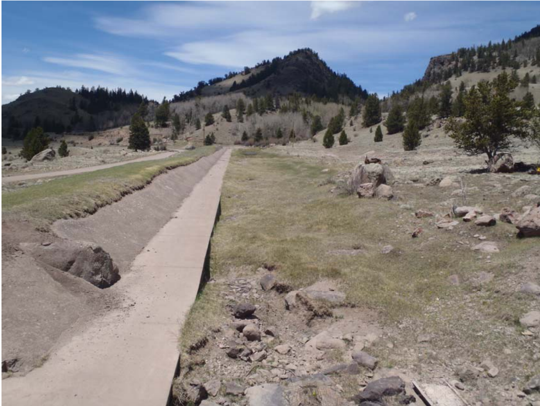
10. Looking upstream along the canal section with the box culvert that conveys winter flow. Slide area in background has caused high seepage rates through the canal section.
