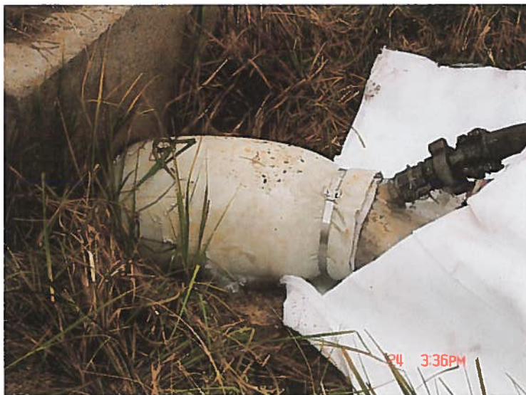
Figure 8 Close up view of the apparatus used to cure the CIPP. Both the inner and outer liner layers used to make the CIPP are visible.
