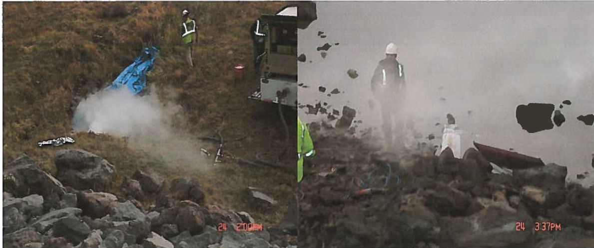
Figure 6 & 7 Steam showing at both ends of the outlet pipe.
