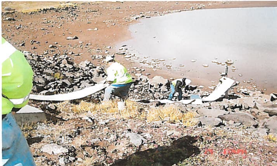
Figure 1 Workers laying out the liner along the inner face of the dam
