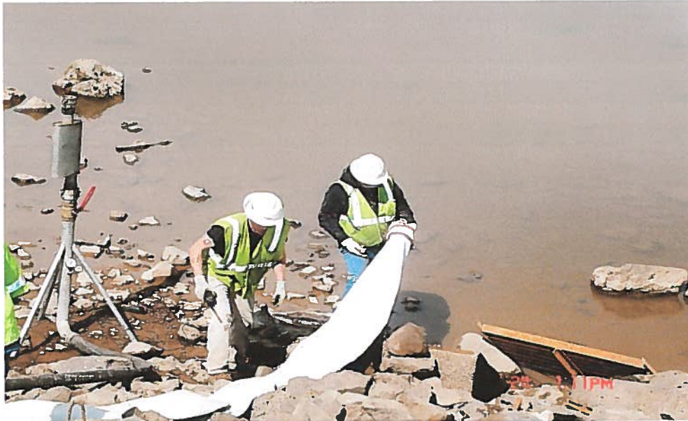
Figure 2 Wrapping a rope around the end of the heavy liner before using the rope to carefully pull the liner through the steel pipe to the exit on the outside of the dam.
