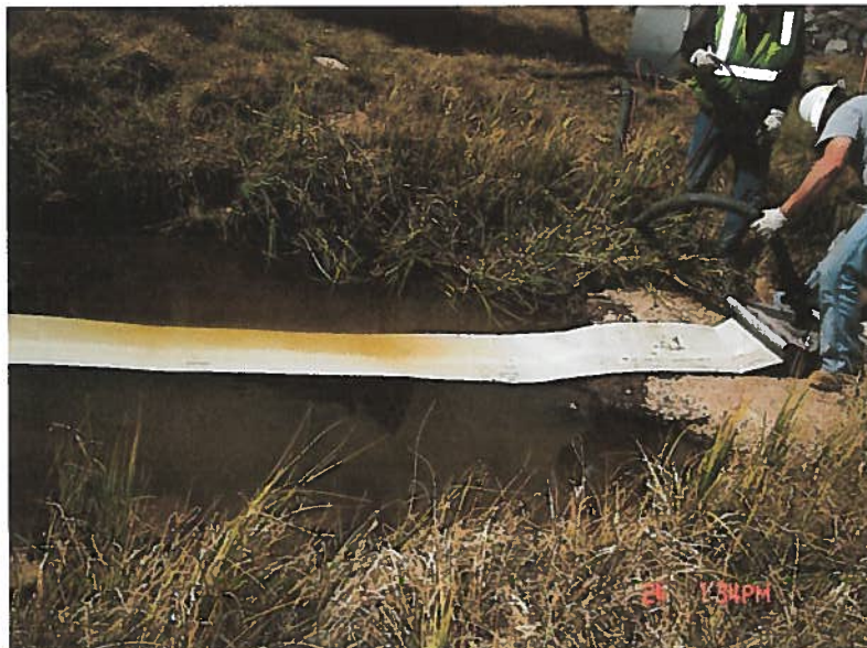
Figure 3 Inner liner going through the rollers. The 2 ½ inch air hose is visible on the far right in the hand of one of the workmen.
