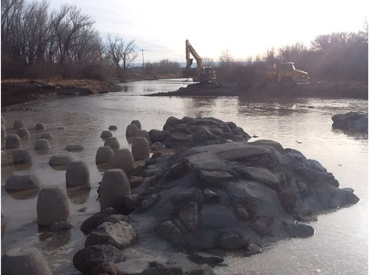
Breaking lower coffer dam – standing on island to left of boat passage.
