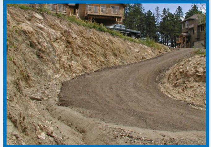
Access roads such as the erosive driveway cut in this photo can be a source of large sediment loads.
