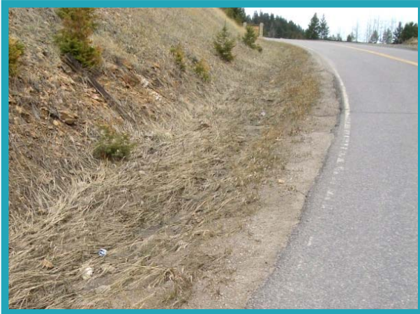
Ditches need maintenance. When ditches fill with sediment, there is no capacity for runoff in the ditch and excess flow can cause scour downstream. ....
