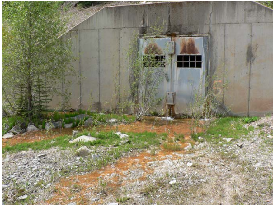
Photo 7.4. The Santa Cruz Mine Adit. This Photo shows the Controlled Flow Channel (left) and the Uncontrolled Flow that is Circumventing the Remedy.
