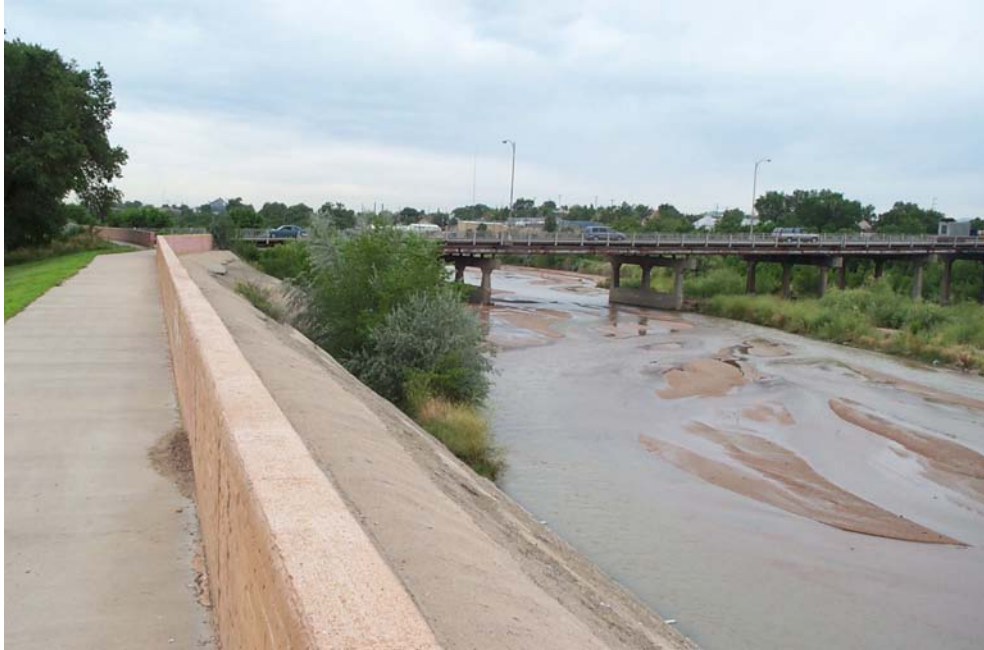
Photo 4-27: Storms drains emptying into Fountain Creek at this location are now several feet under the typical creek level due to aggradation of the channel bed with sediment creating a maintenance problem for the City of Pueblo (note flood control dike at left in photo).
