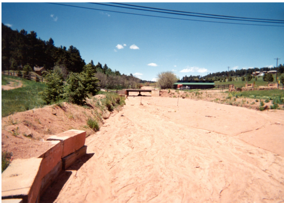
Photo 4-4: Channel sediment aggrading in the channel below the bridge connecting to the Old Crystola Road downstream of Woodland Park.
