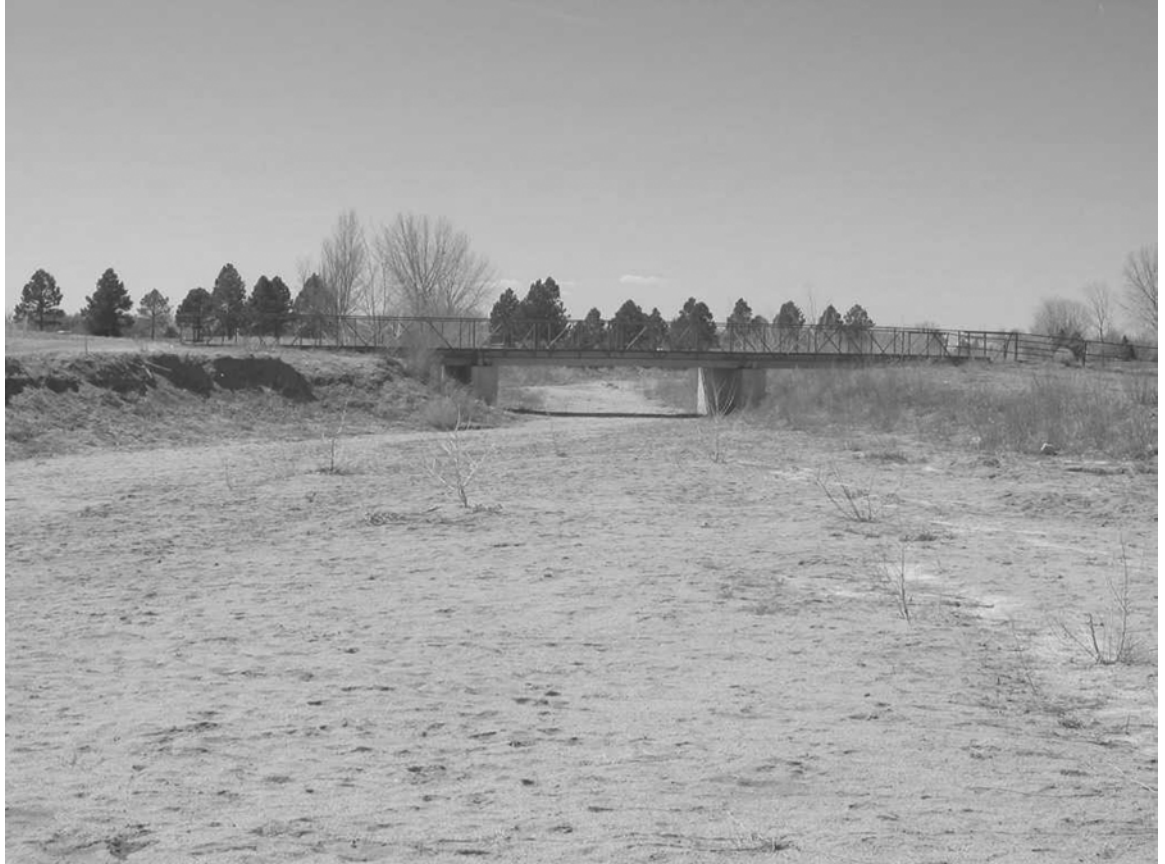
Photo 4-23: A view looking downstream on Jimmy Camp Creek at the pedestrian bridge where the upper end of berms confine stream flow in Jimmy Camp Creek to a narrow corridor, leaving the floodplain mostly cut off from the channel.
