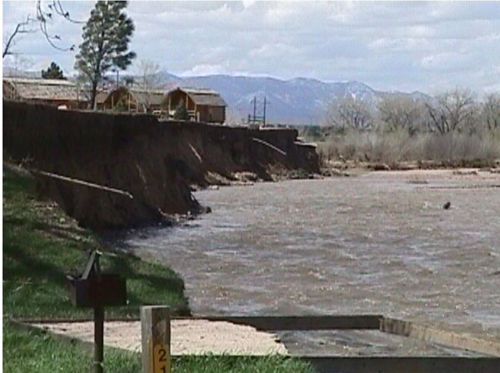
Photo 4-20: Erosion of the Fountain Creek bank during the flood of 1999 adjacent to the KOA campground.
