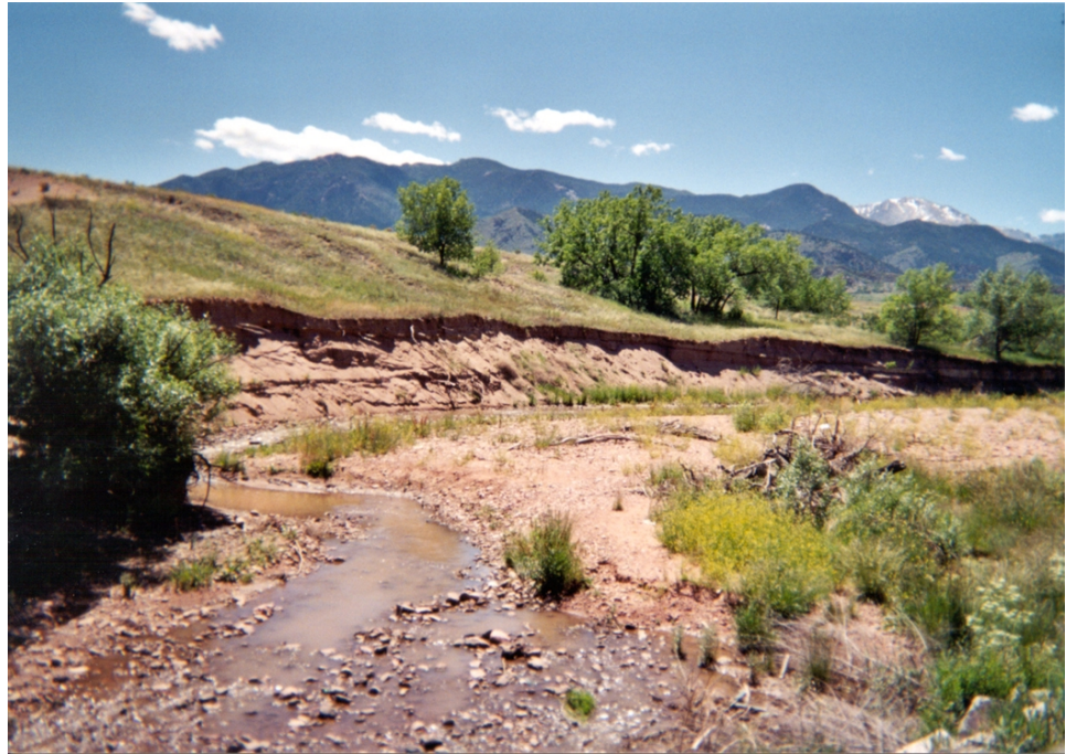
Photo 4-7: Erosion in the bank of Fountain Creek upstream of the Monument Creek confluence.
