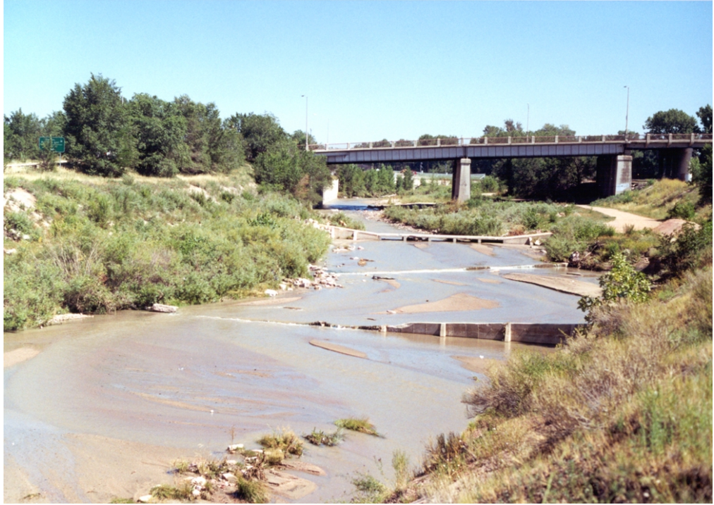
Photo 4-11: Old concrete check structures in the lower Monument Creek channel are ineffective and have been damaged as a result of channel changes and flooding. Newer grouted riffle drop structures seen in Photo 4 – 14 have replaced the concrete check structures.
