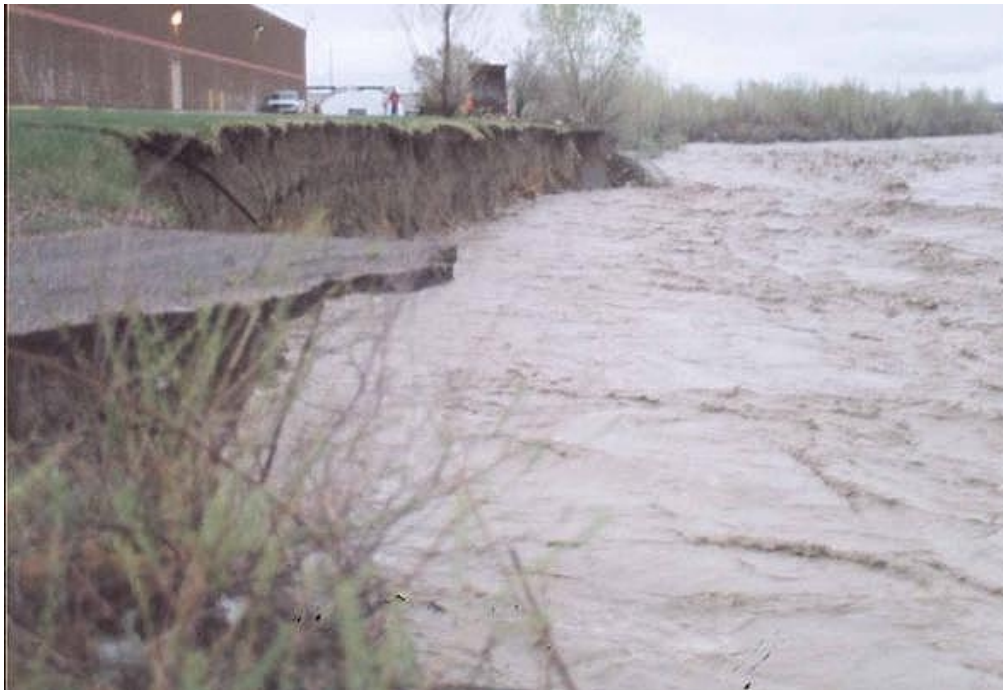
Photo 4-28: View of the embankment adjacent to the Target Store that had to be closed due to heavy flooding. Flooding caused heavy bank erosion, destruction of the gabion protection, and eventually exposed the foundation.
