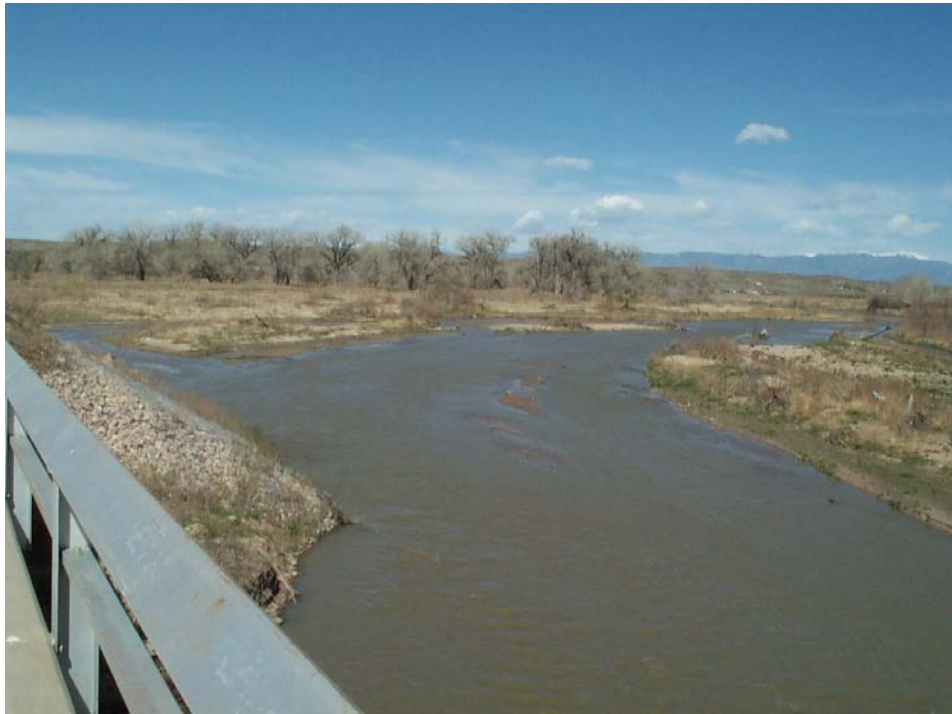
Photo 4-29: View from Pinon Bridge showing Fountain Creek flow directed toward the bridge abutment, thus suggesting that erosion and stability will be a continued problem in future floods.
