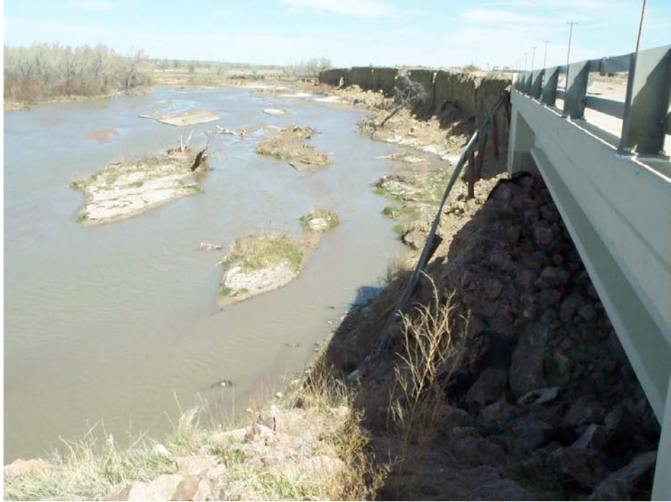
Photo 4-30: Bank erosion and bridge damage after the 1999 flood, which continues today at the Overton Road site.
