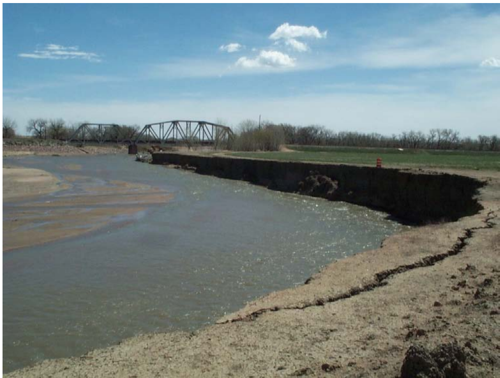
Photo 4-21: Meander migration and erosion of the outside stream bank of Fountain Creek upstream of the Old Pueblo Highway Bridge is causing loss of agricultural land.
