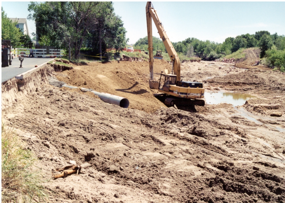
Photo 4-12: An intense thunderstorm during the summer of 2001 caused bank erosion damage on Cottonwood Creek at the Epernay Apartments.
