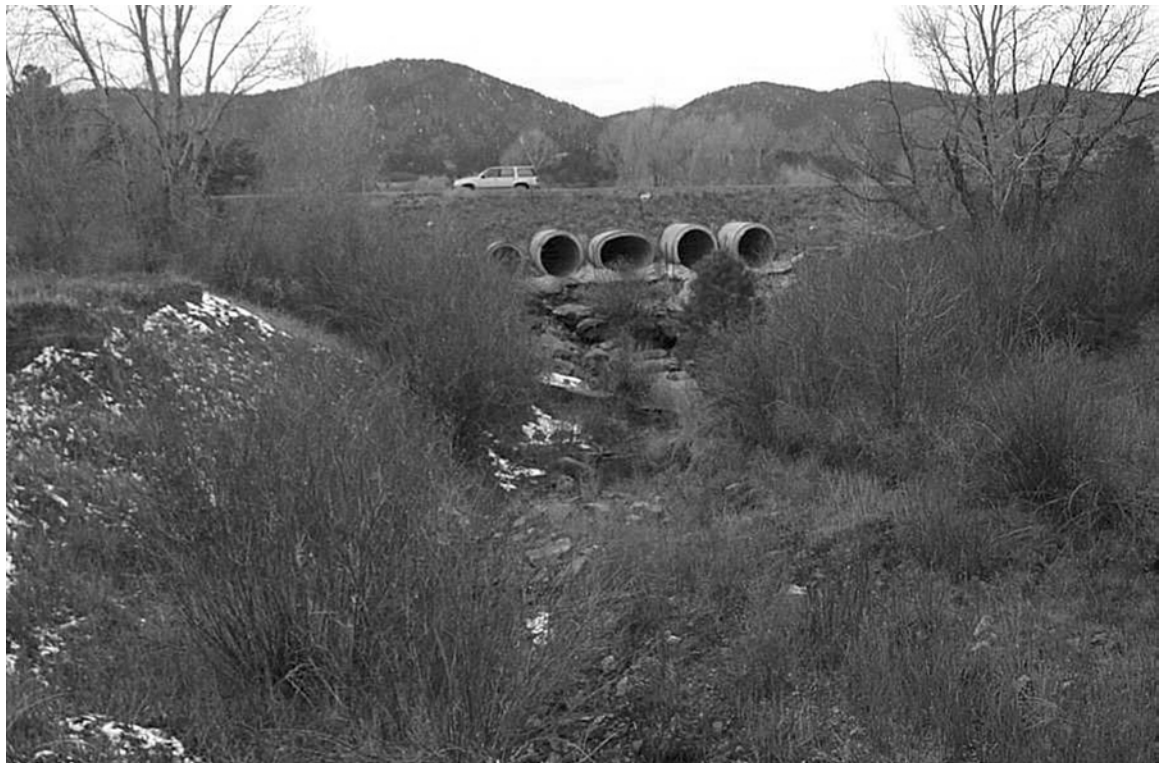
Photo 4-16 An upstream view of Red Rock Ranch Drive and the Monument Creek channel immediately downstream of the stream underpass. The channel has degraded 15 to 20 feet below the original rechannelized grade.
