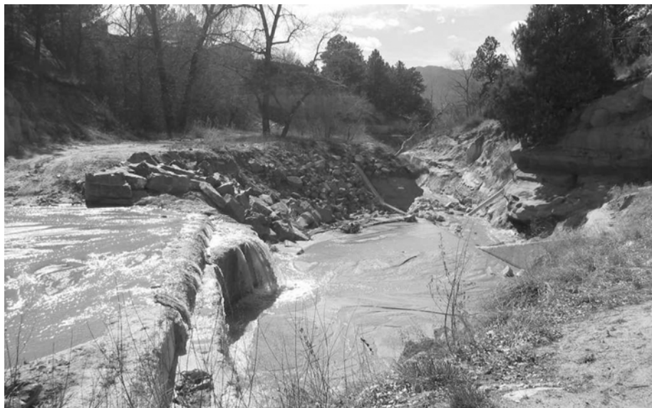
Photo 4-18: Two relatively old drop structures control channel degradation on Cottonwood Creek midway between Academy Boulevard and I-25. The concrete drop in the foreground encases a pipeline. Both drops show signs of undercutting of the bedrock on which they are founded. Enhancement of these structures may be needed to prevent failure and massive erosion of the upstream channel.
