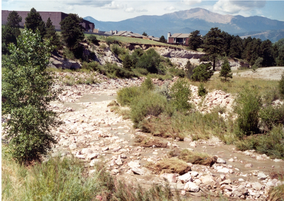
Photo 4-13: Channel bed degradation on Cottonwood Creek downstream of Academy Boulevard. Riprap has been placed in attempts to control erosion.
