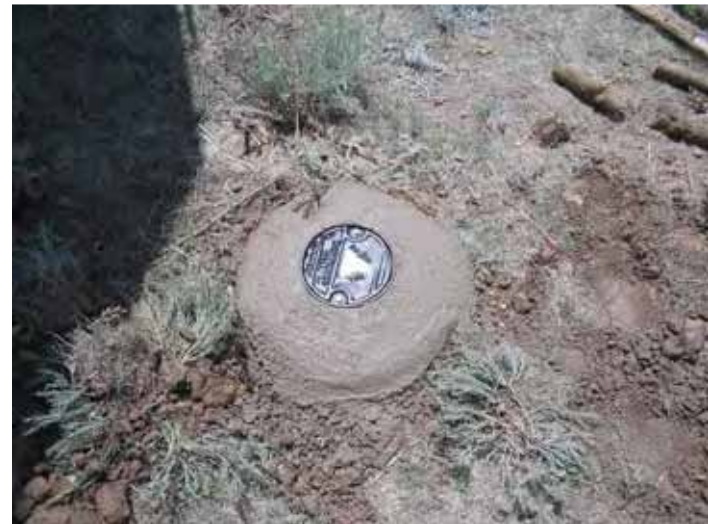
Piezometer with flush mount cover
